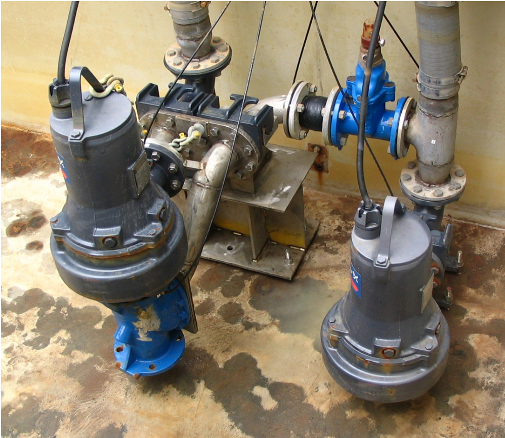
Figure 4.1 Prototype pumps installed in test tank.
