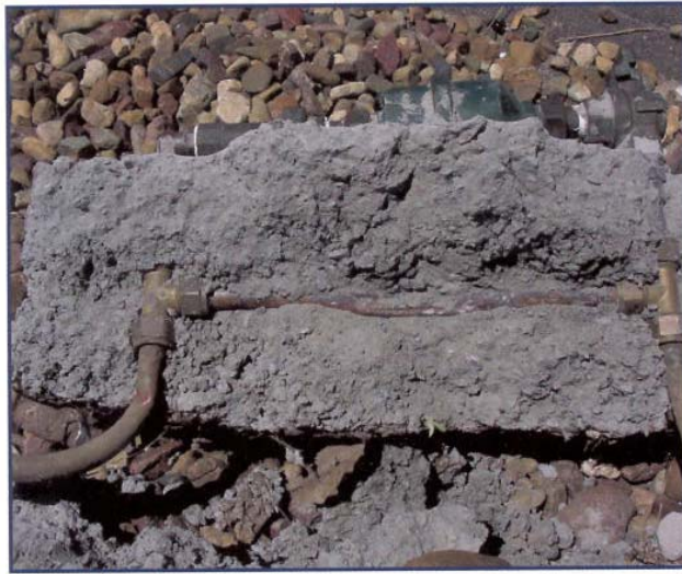
Figure 2.8(b) The illegal meter bypass encased in concrete (Queensland Environmental Protection Agency and Wide Bay Water Corporation, 2005).
