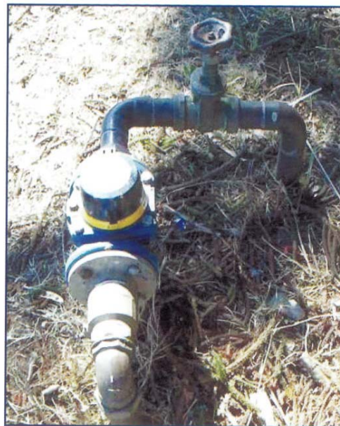
Figure 2.5 (b) Unnecessary bends around the water meter (Queensland Environmental Protection Agency and Wide Bay Water Corporation, 2005).
