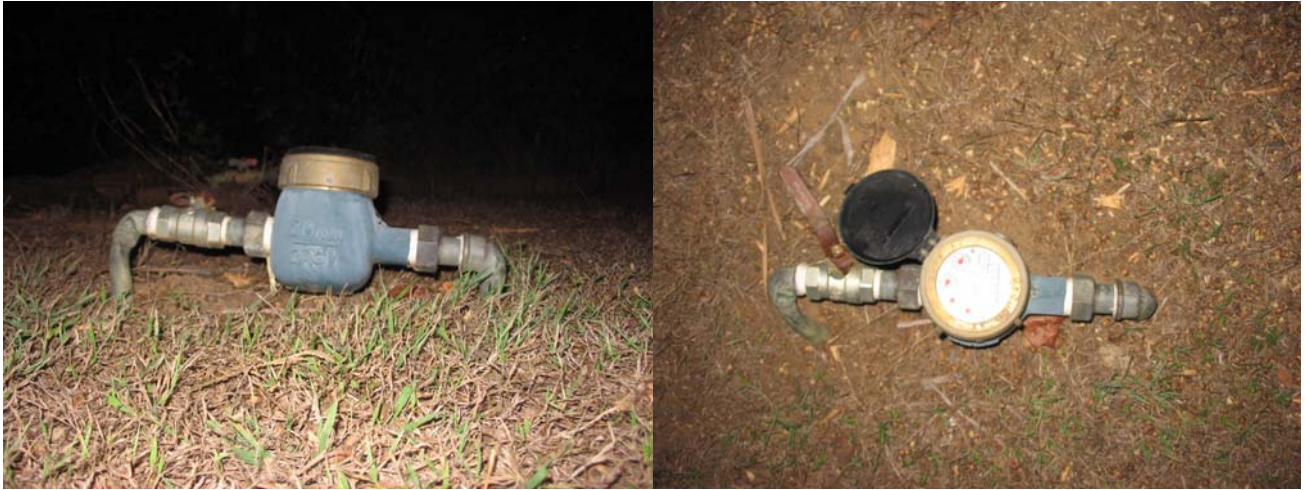
Figure 2.5(a) Incorrect installation of an above ground water meter (Chris Martin, 2007)
