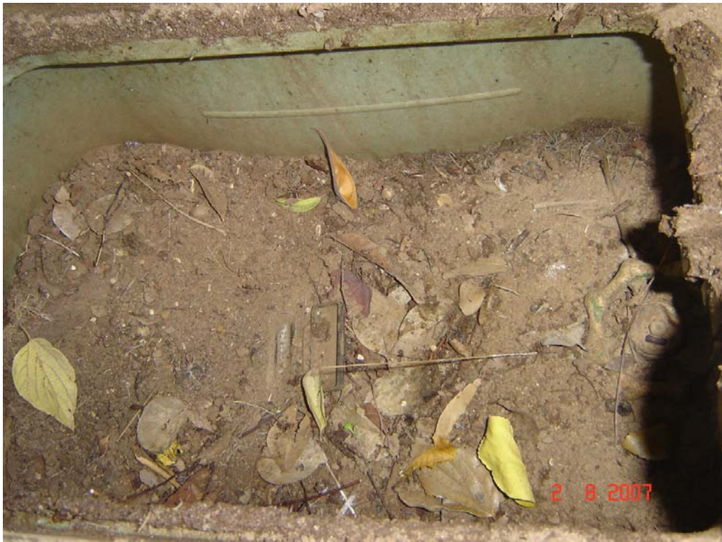
Figure C5 Silt/Soil covering the entire water meter
