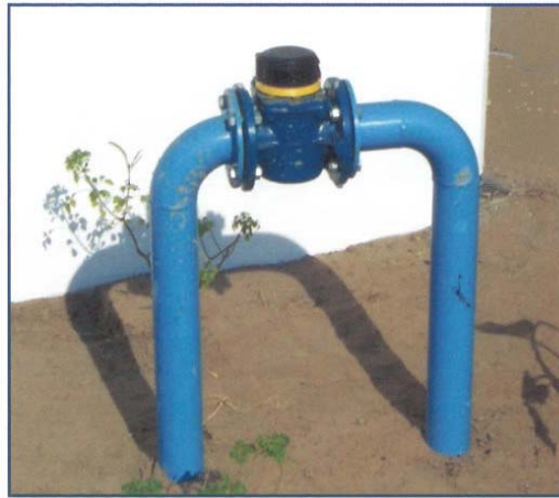
Figure 2.7 This installation is almost certain to result in trapped air causing air surges (Queensland Environmental Protection Agency and Wide Bay Water Corporation, 2005).
