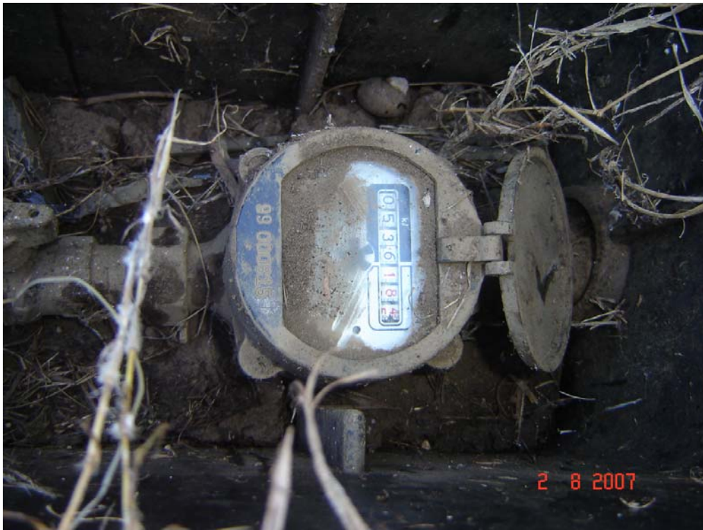
Figure C1 Silt covering the consumption volume on the water meter
