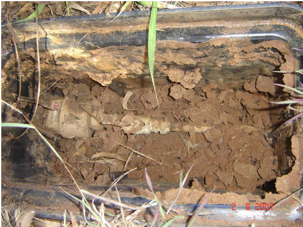
Figure C8 Ant nest within the water meter box
