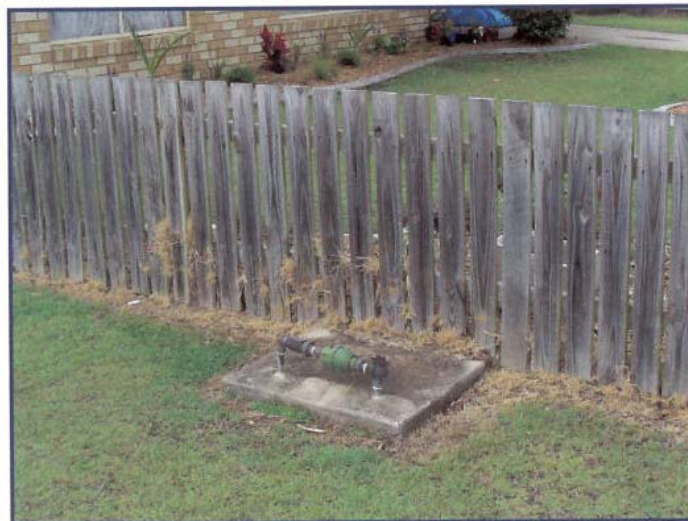
Figure 2.8(a) A bypass is cleverly concealed within a concrete slab (Queensland Environmental Protection Agency and Wide Bay Water Corporation, 2005).
