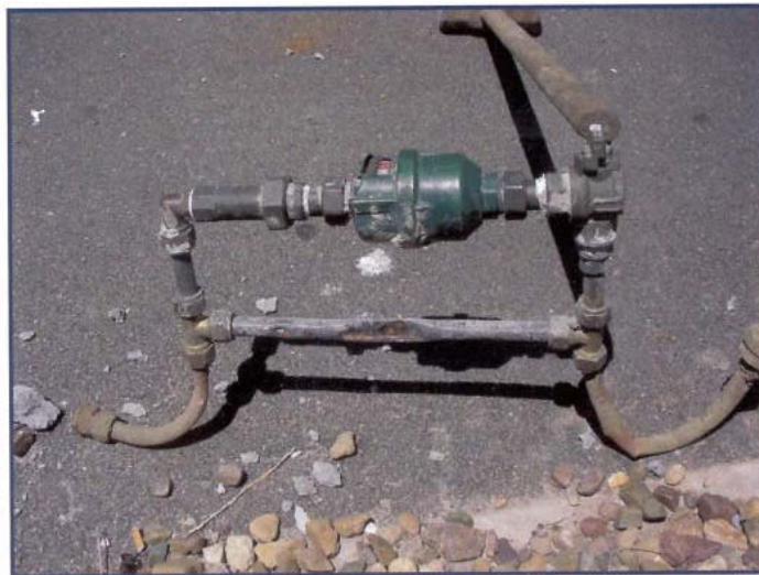
Figure 2.8(c) The illegal domestic meter bypass (Queensland Environmental Protection Agency and Wide Bay Water Corporation, 2005).
