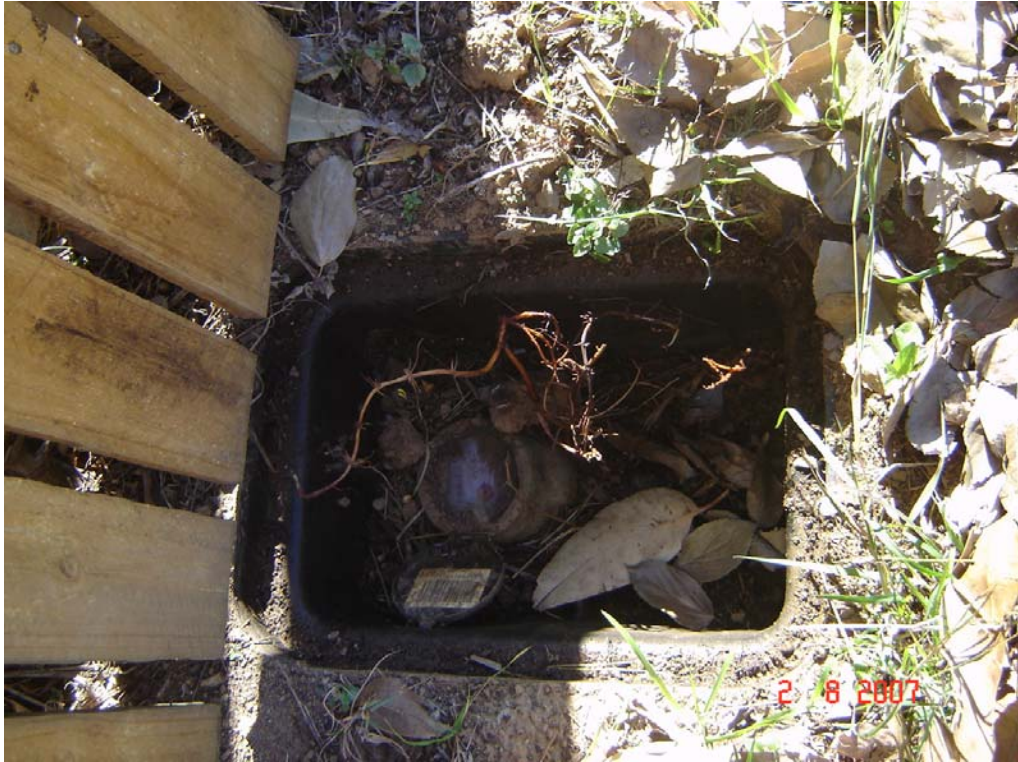
Figure C3 Fence lines on properties built up to or over the water meter
