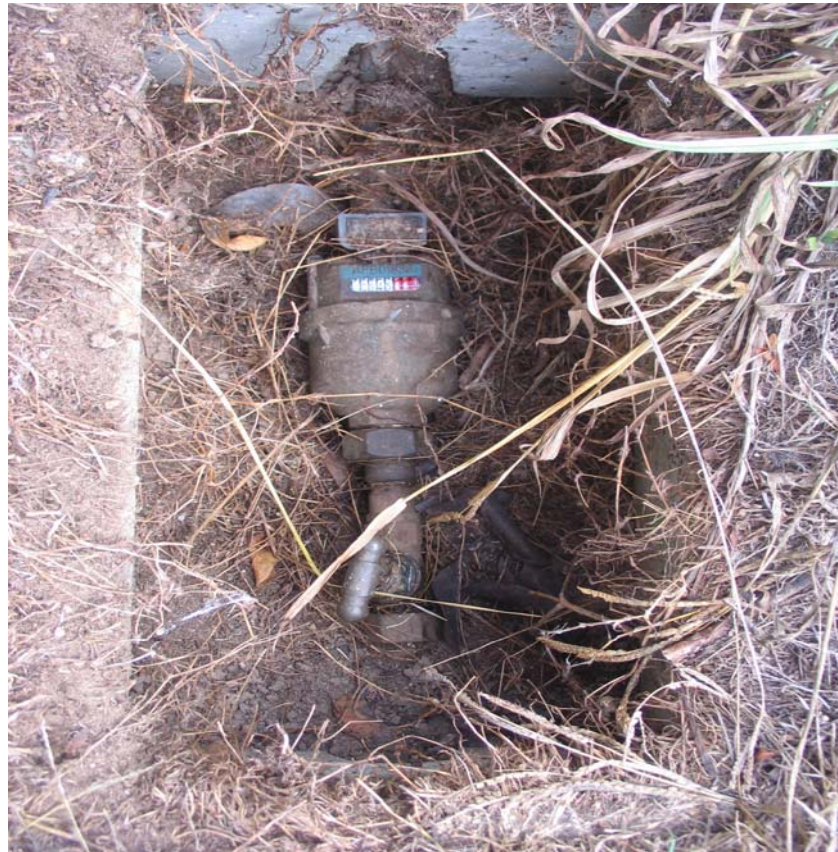
Figure 2.1 A Typical Residential QLD Water Meter (Chris Martin, 2007)
