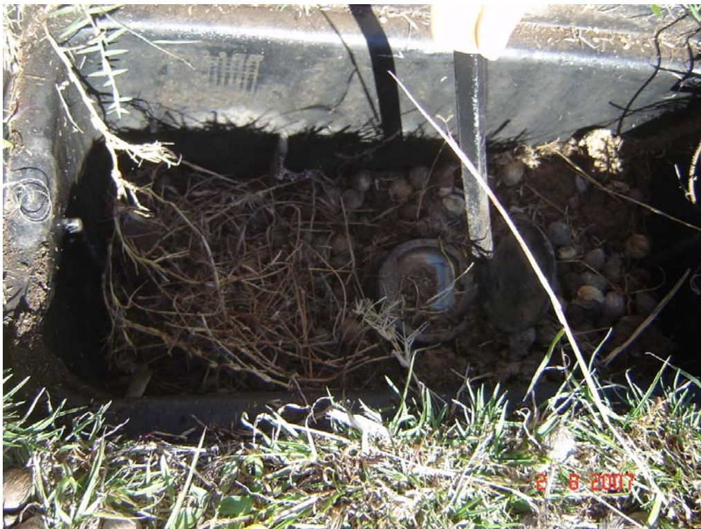
Figure C2 Water meter full of debris (Seeds, grass and soil)
