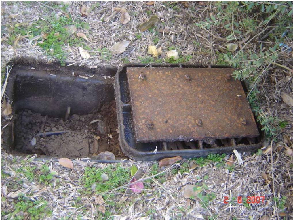
Figure C6 Property owners tampering with the water meter
