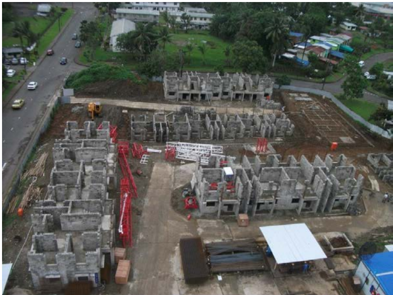
Figure 21: Shows an Overall Photograph of the Site during Construction Works in 2012 (NRW Macallan)
