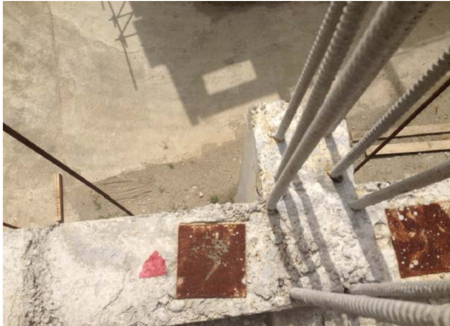
Figure 24: Showing Almost Zero Cover to Main Bar (NRW Macallan)
