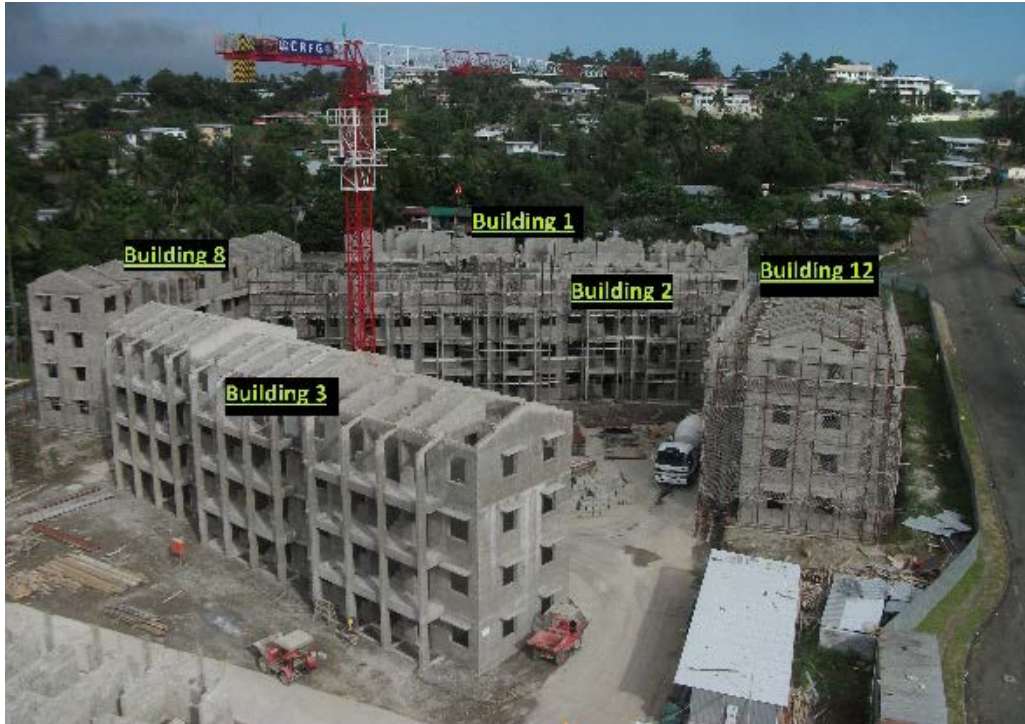
Figure 22: Shows an Overall Photograph of the Site during Construction Works in 2013 (NRW Macallan)
