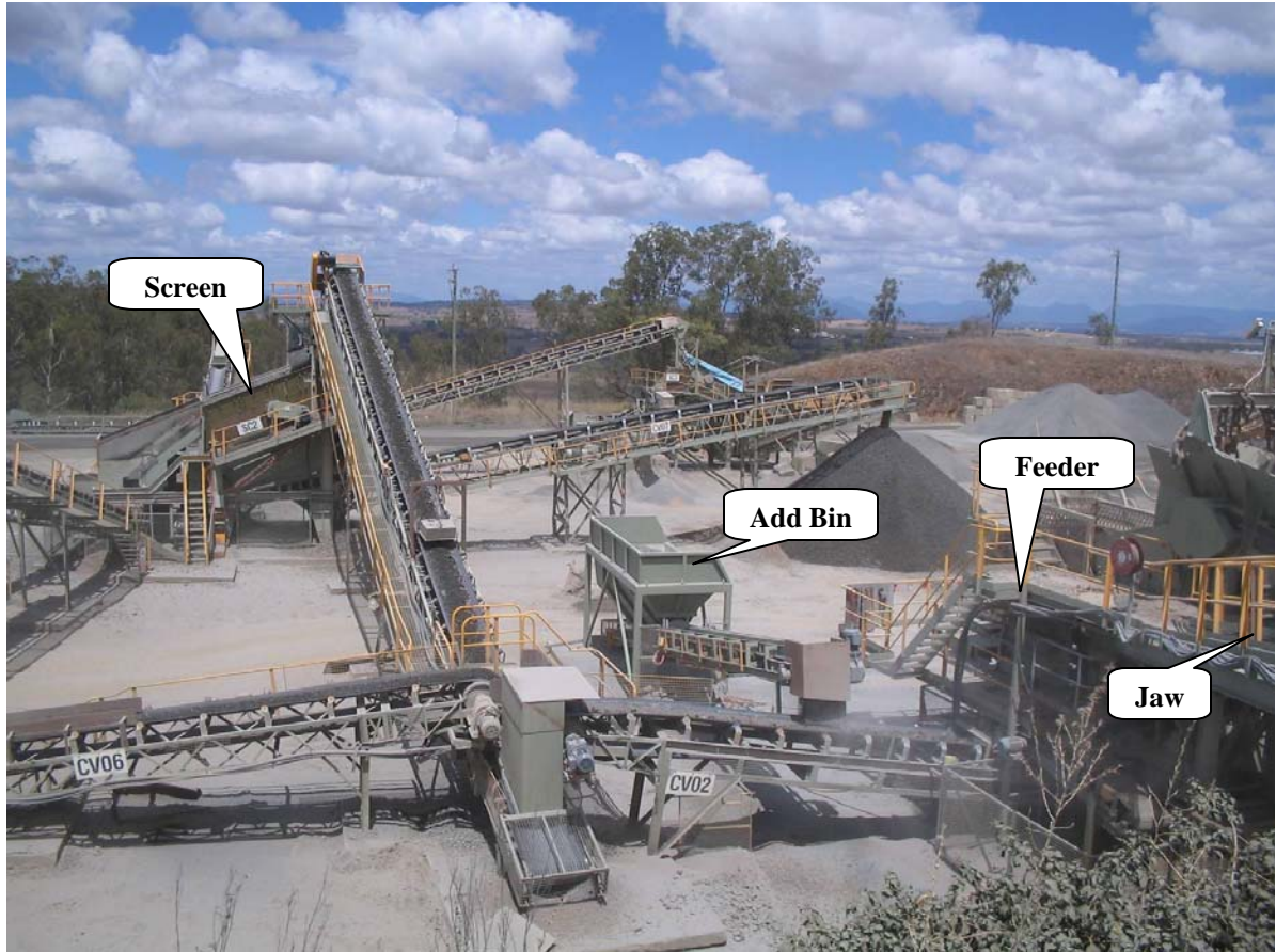
Figure 2.2 – Picture of Purga Crushing Plant 1 taken from the control box
