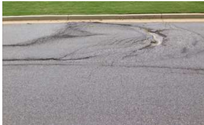
Figure 2.5: Crescent shaped crack (Grover Allen, 2017)
