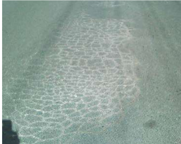
Figure 2.6: Crocodile Cracking (TMR, 2017)
