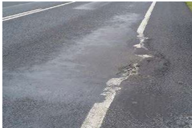
Figure 2.3: Pavement shoving (TMR, 2017)
