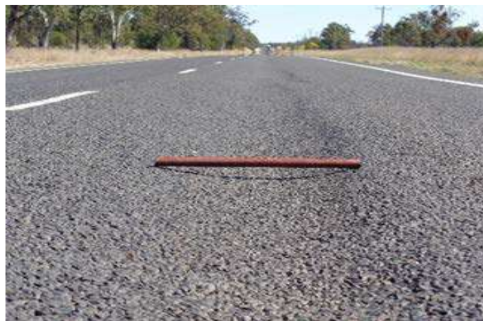
Figure 2.2: Pavement rutting (TMR, 2017)
