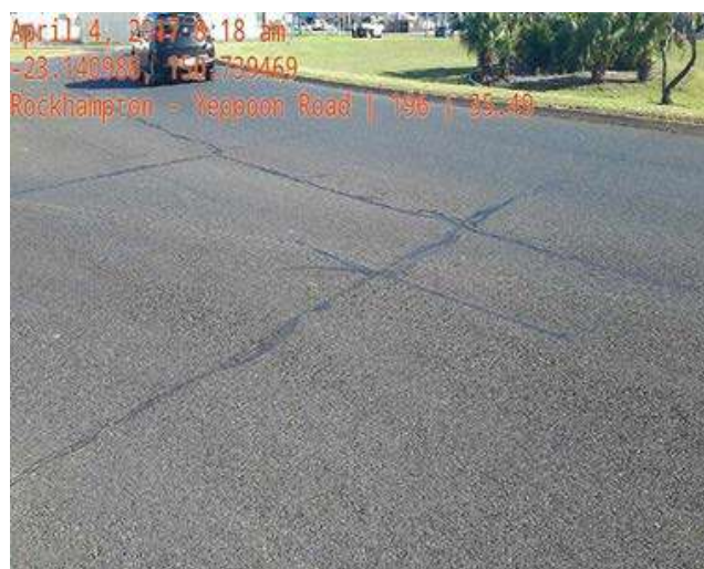
Figure 2.4: Block Cracks (TMR, 2017)
