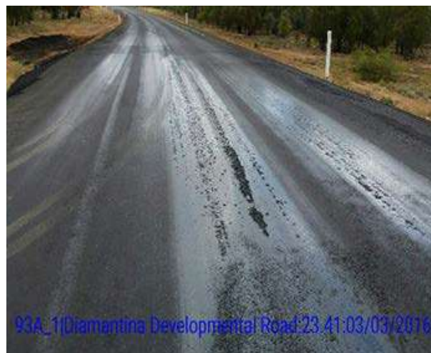
Figure 2.11: Flushing, Bleeding seal (TMR, 2017)
