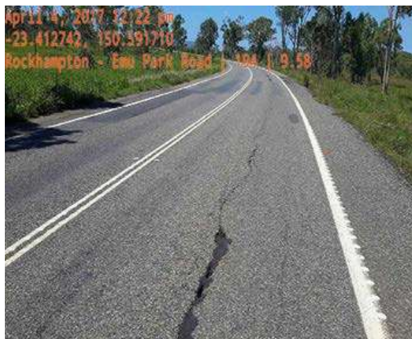
Figure 2.7: Longitudinal cracks (TMR, 2017)
