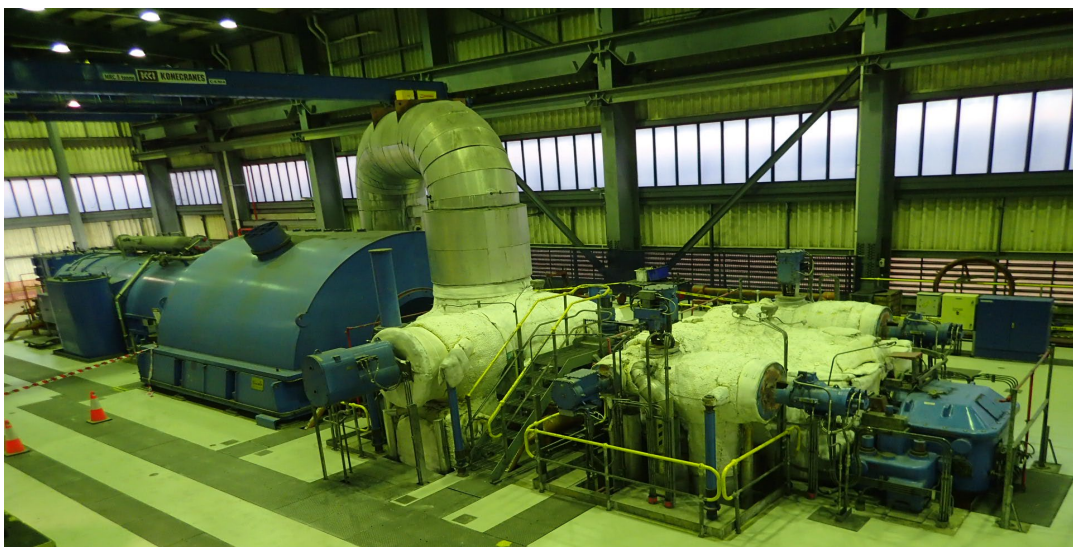
Figure 1.3 Collie Power Station Turbine Generator
