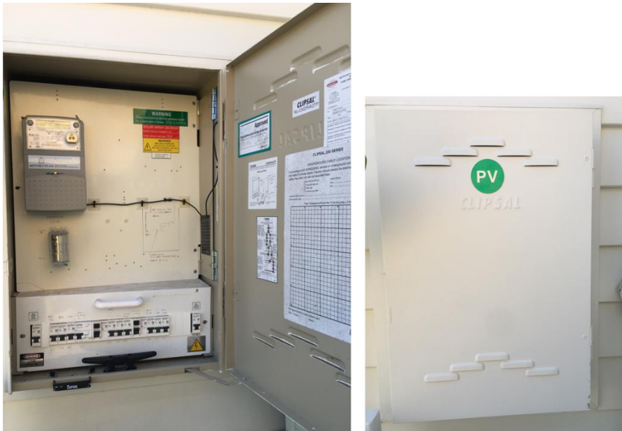
Figure B1.9.9: Main switch board with incorporate advance isolation system for safety.
