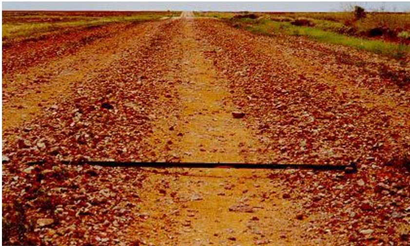
Figure 7 (Austroads Ltd., 2018, p. 54) Dry Rutting on Unsealed Roads
