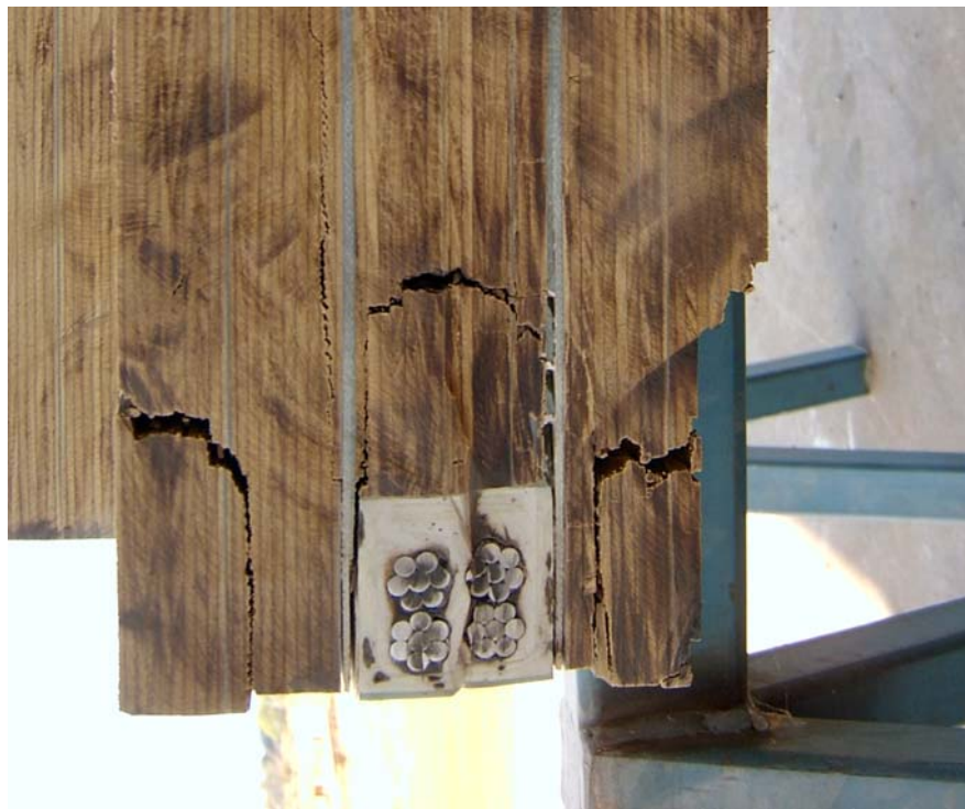
Figure 6.9 Extent of LVL cracking through beam section
