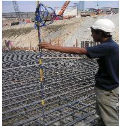
Figure 5.6: Prior to installation, the thermocouple wires were tied to additional steel bars.
