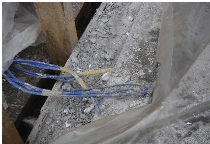
Figure 5.2: Concrete is protected by a layer of plastic sheets to prevent lost of water during curing stage.
