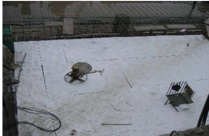
Figure 5.1: Concrete temporary covered by polyethylene sheeting on the plastic sheets to protect from the Sun.
