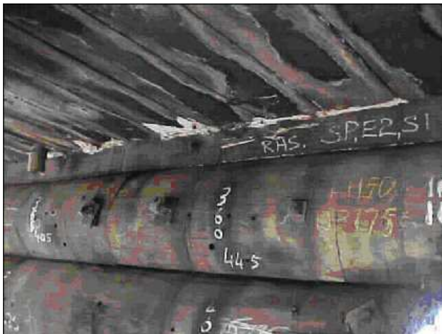
Figure 1.1: White Rot Degradation of Frank Creek Bridge, Wide Bay District (Source: [3])
