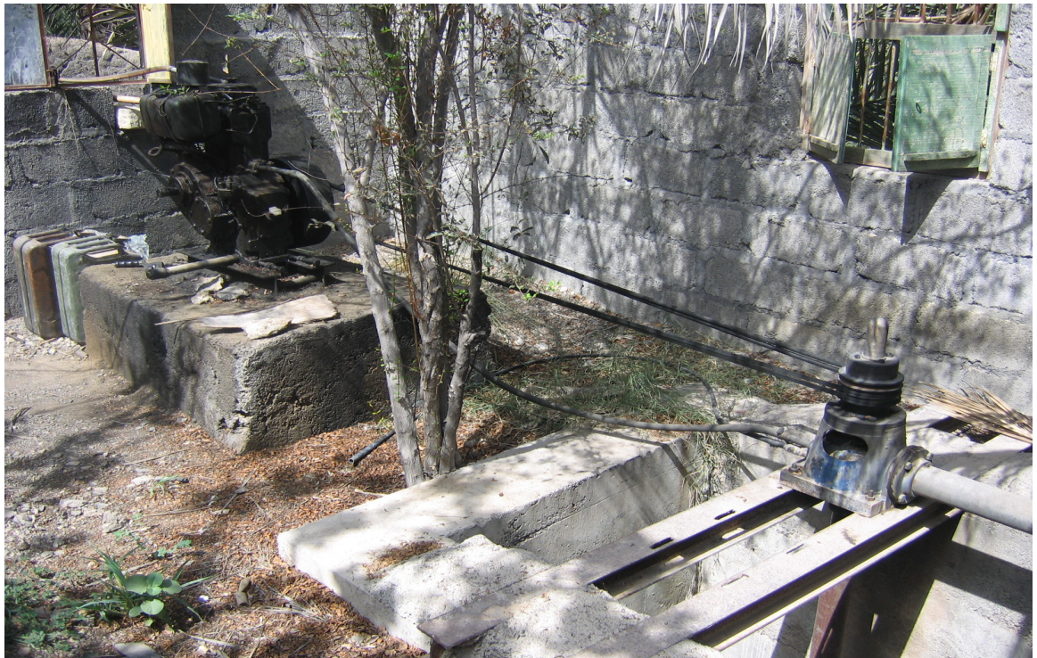
Figure 3.2: The diesel pumping system widely used in Oman.
