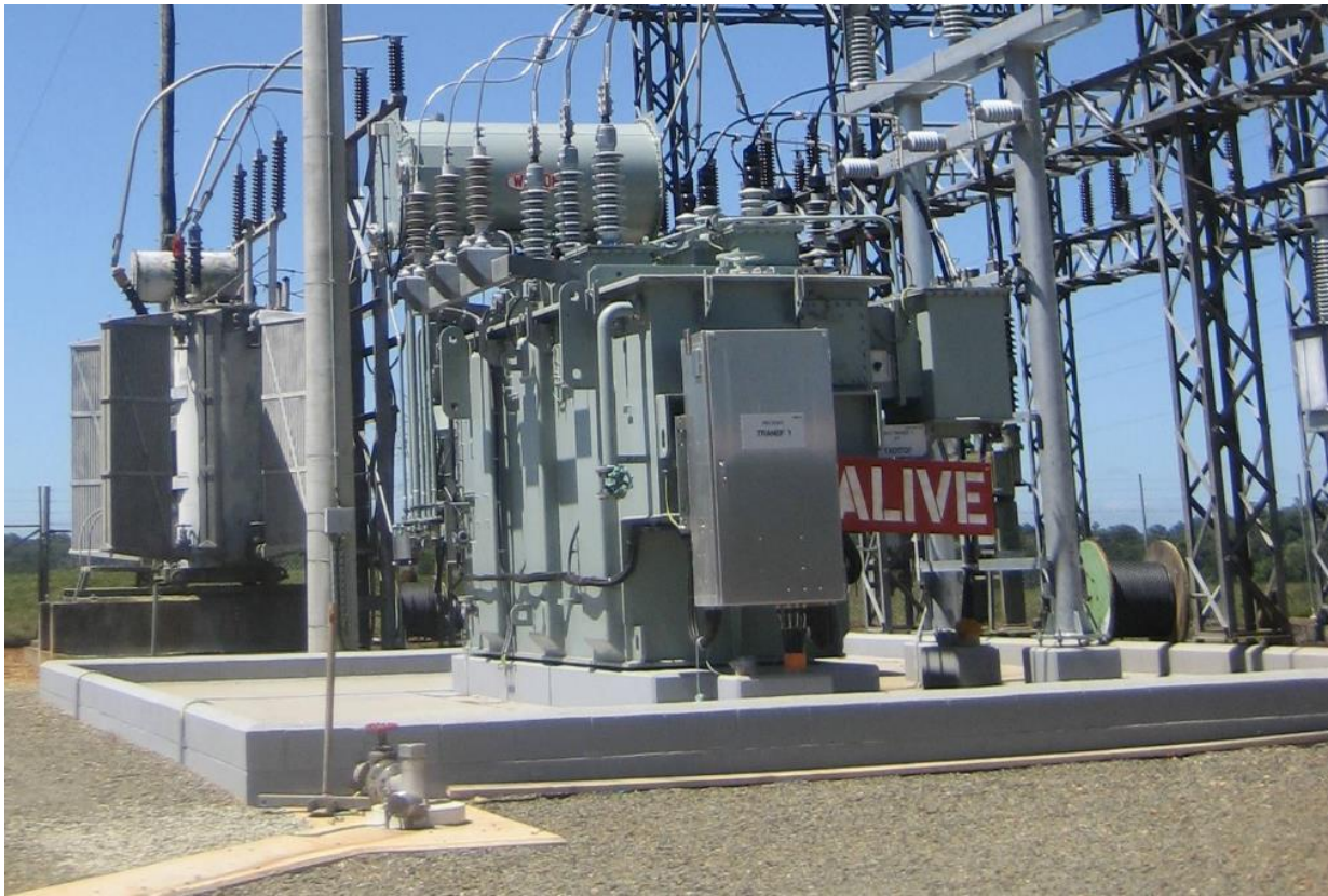
Figure 1.2: Transformer bund, Evelyn Substation.
