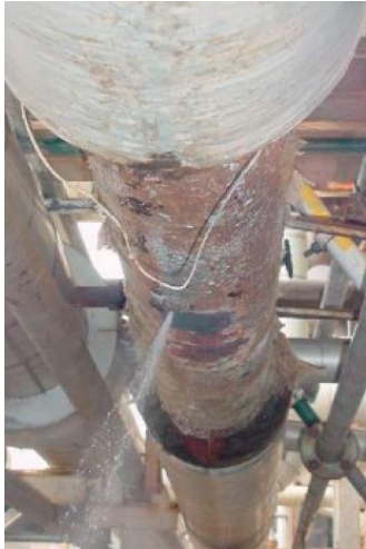
Figure 2.33: CUI of carbon steel pipe (Winnik 2015)
