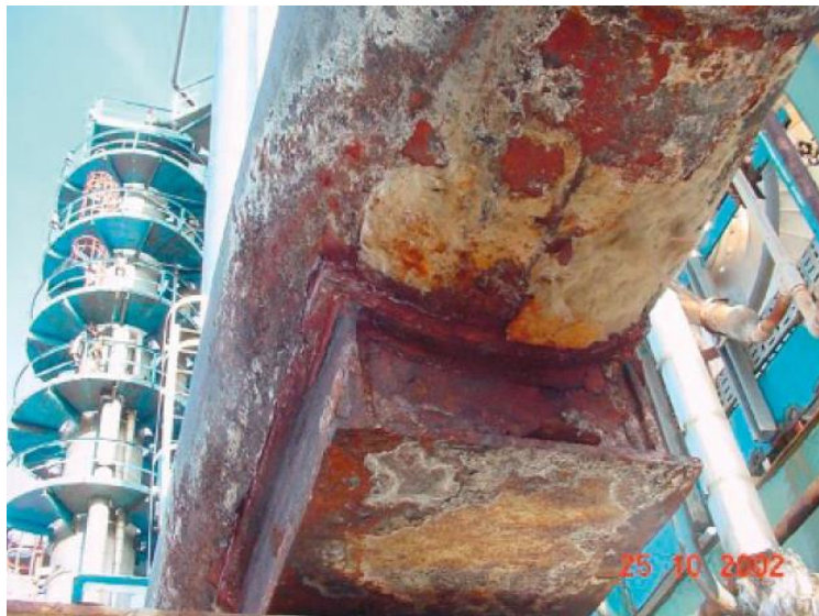
Figure 2.34: CUI of carbon steel pipe support (Winnik 2015)
