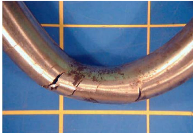
Figure 2.32: Type 304 stainless steel cracking under insulation (American Petroleum Institute 2011)
