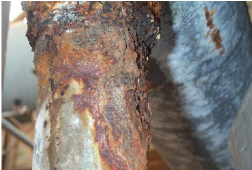
Figure 2.36: CUI of Tee section insulated carbon steel piping after removal of insulation (American Petroleum Institute 2011)
