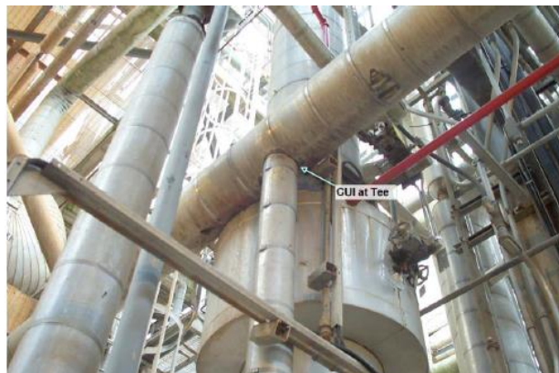
Figure 2.35: Tee section insulated carbon steel piping before removal of insulation (American Petroleum Institute 2011)
