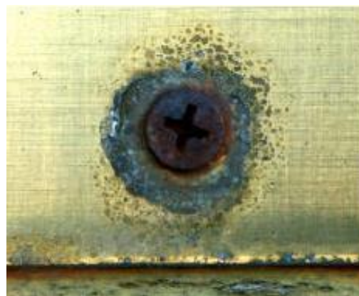
Figure 2.14: Sample of galvanic corrosion (Galvanic corrosion 2021)
