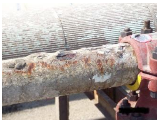
Figure 2.22: An LPG line suffered atmospheric corrosion (American Petroleum Institute 2011)
