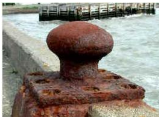
Figure 2.8: Result of uniform Corrosion (Uniform corrosion 2021)
