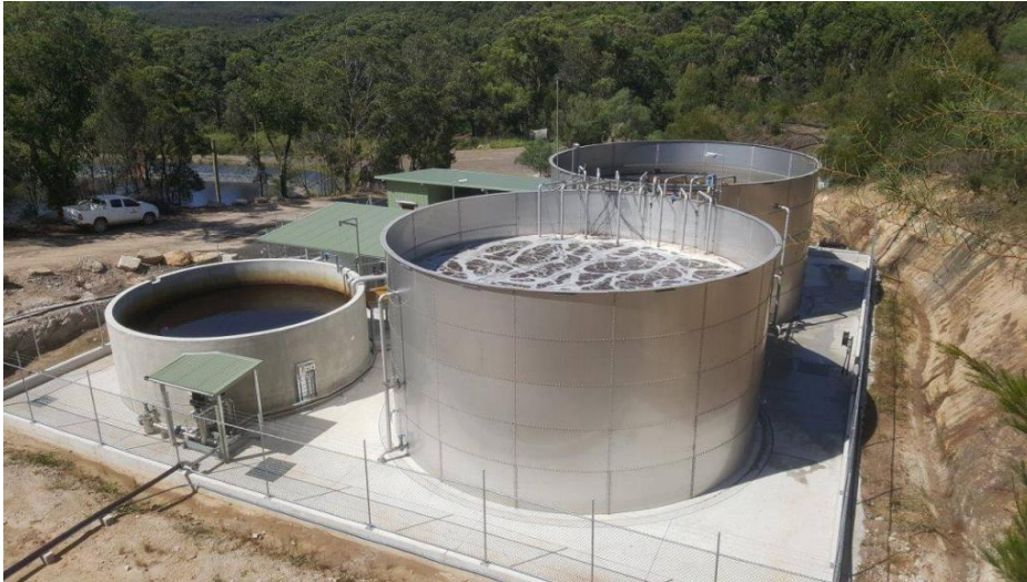
Figure 6. Stainless steel tanks at the Kimbrikki installation. (Kimbrikki news, 2019)
