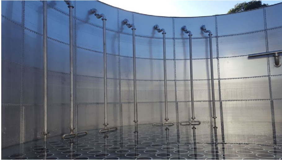
Figure 7. Lucas Heights stainless steel tank. (JPG Engineering, 2019)
