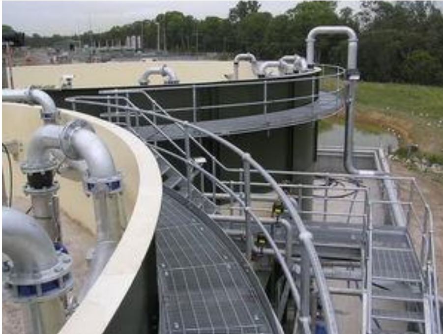
Figure 8. Landfill leachate treatment facility at Eastern Creek, Sydney. This plant uses ammonia oxidation to treat its leachate. (JPG Engineering, 2019)
