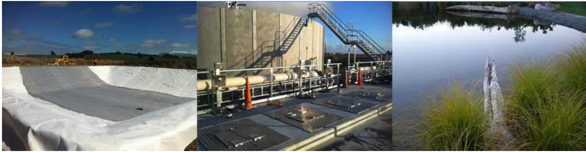
Figure 5. Example of liner for leachate dam, processing tanks and operational dam at Hampton Downs Landfill - North Waikato (IS Dam Lining, 2021)
