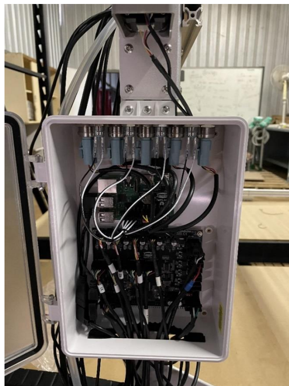
Figure 7: The completed FarmBot Electronics Box.
