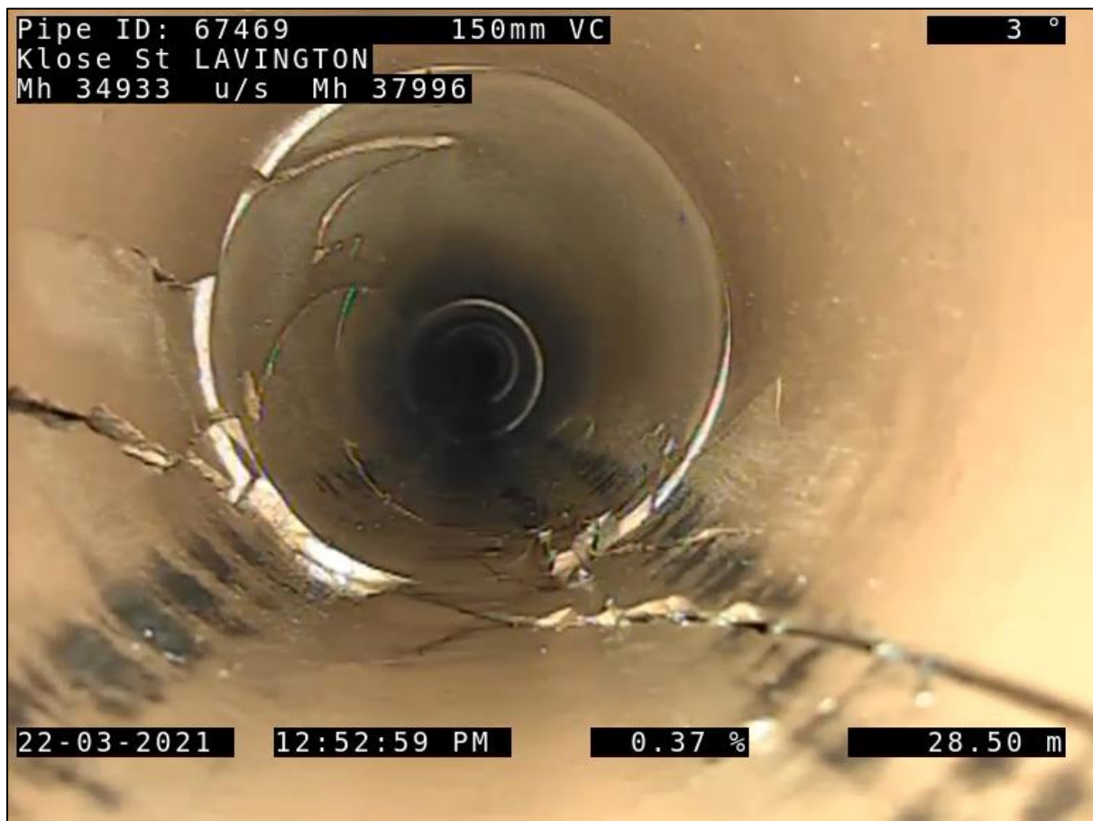
Figure 3.4: Sewer Inspection Image with cracking (Albury City Council Sewer Inspection Program, 2021)
