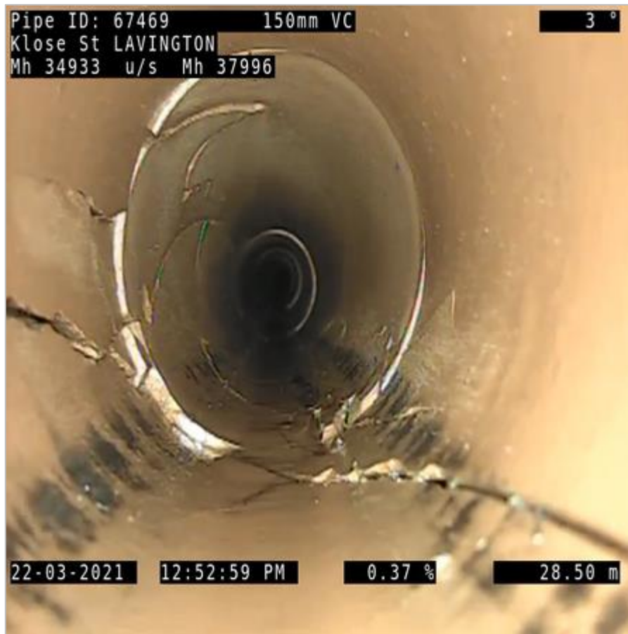
Figure 3.5: Sewer Inspection Image with cracking (resized) (Albury City Council Sewer Inspection Program, 2021)
