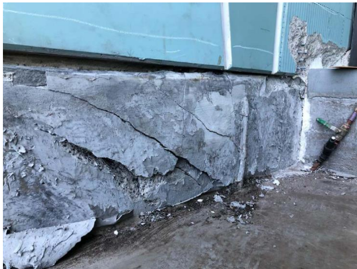
Figure 2.1: An example of a damaged hob beam - Opal Tower
