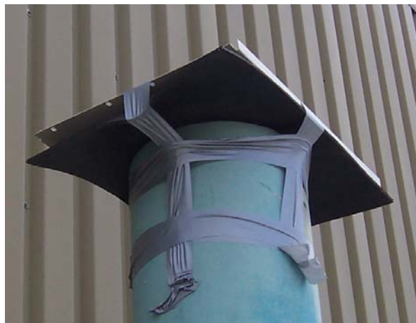
Figure 16 - Air Extraction Turbine Roof Discharge Cap
