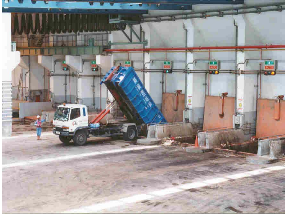
Figure 1.3.1.2: Overview of Refuse Truck Discharged Refuse into the Refuse Bunker
