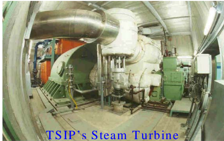
Figure 1.3.5.4: Overview of turbine room that steam turbine drives a generator to produce electricity.
