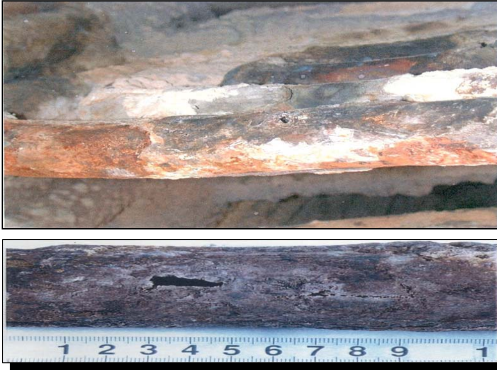
Figure 3.5.3 B: Effect of corrosion on the super heater tube
