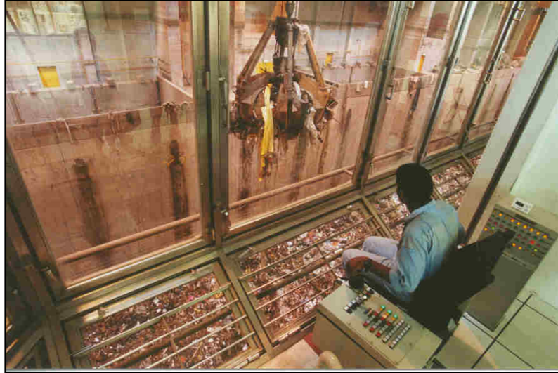
Figure 1.3.1.4 a: Operator control the overhead grab cranes to feed the refuse into the Charging Hopper
