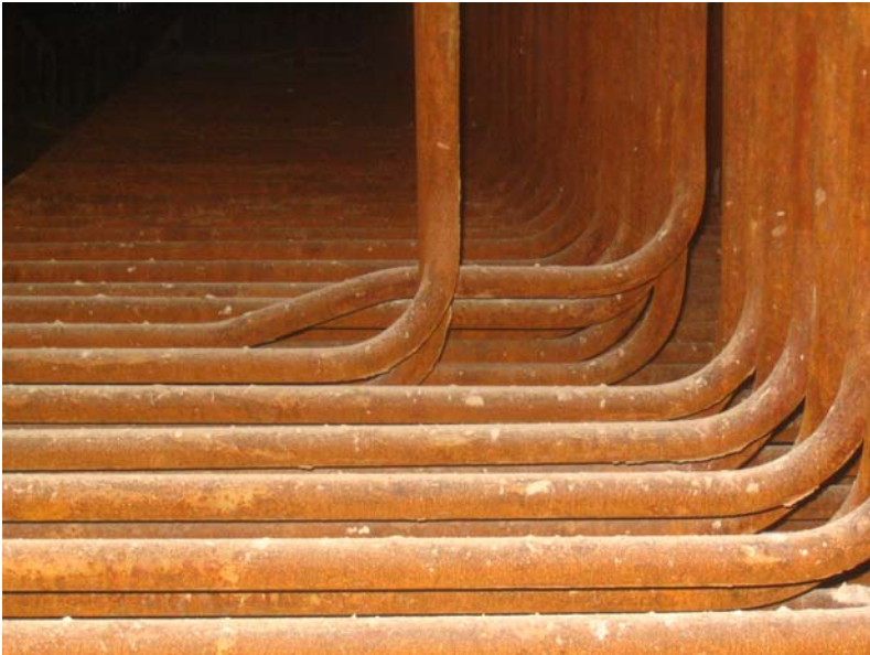
Picture 4.3.2.6 : Tubes surface before and after cleaning of deposits.
