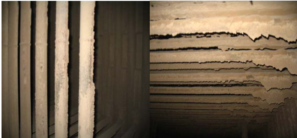
Figure 3.5.3.C Scaling on tubes surface in the third zone before the deposits were cleaned.
