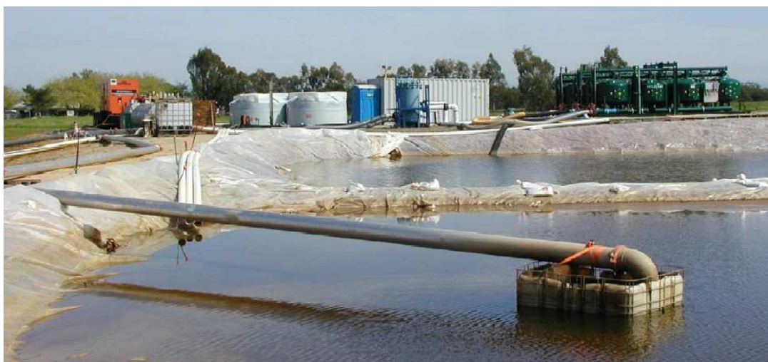
Figure 2.14 Two Clear Creek Systems - Chitosan-Enhanced Sand Filtration Systems treating contaminated runoff at West Park in Roseville, California ( www.clearcreeksystems.com , 2005)
