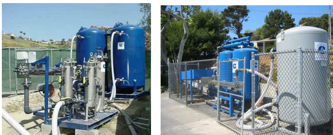
Figure 2.15 Clear Creek Systems – Urban runoff treatment plants utilising modified clay and activated carbon filter media ( www.clearcreeksystems.com , 2005)
