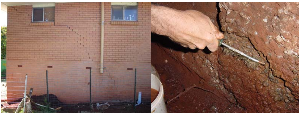
Figure 1.1 Failed foundation step.
