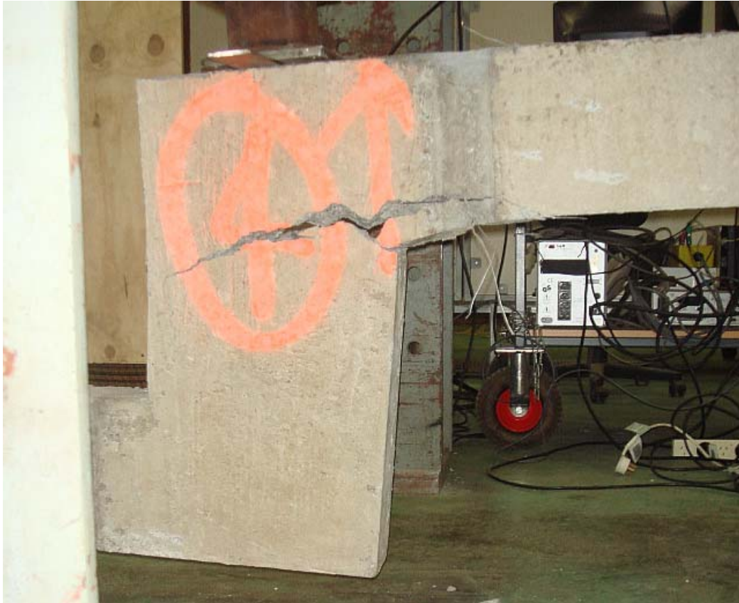
Figure 4.10 Beam 4 crack patterns.
