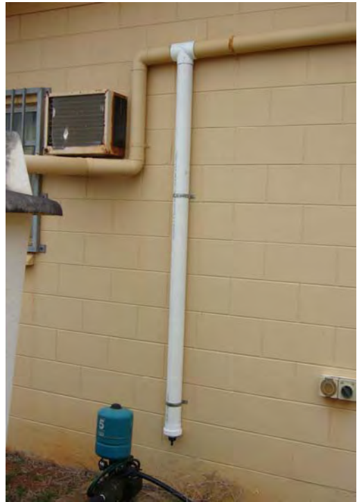
Figure 4.3 First Flush Device - Western
