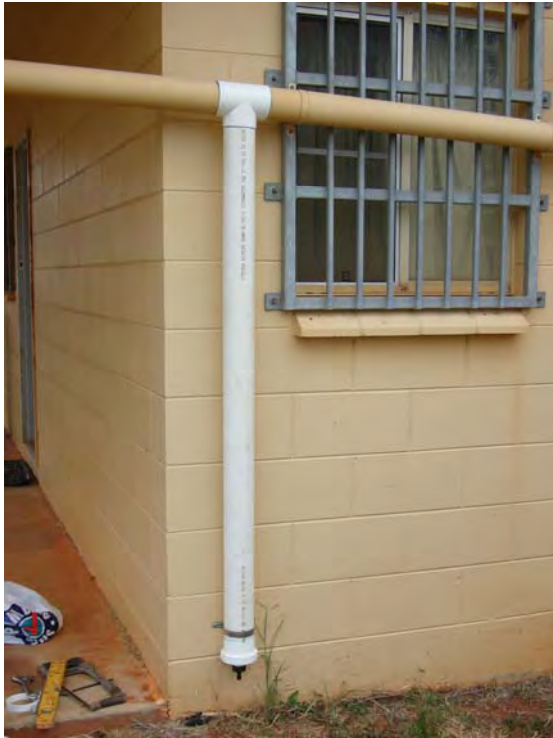
Figure 4.2 First Flush Device - Eastern
