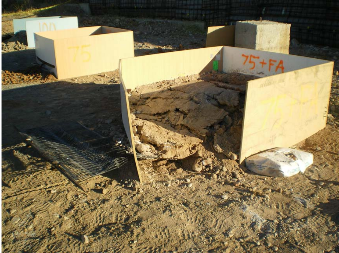
Figure 18 Tensar Geogrid interaction fails under pullout load
