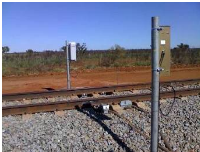
Figure 4.2 Operational ARGUS system track side components. (Inspired Systems)
