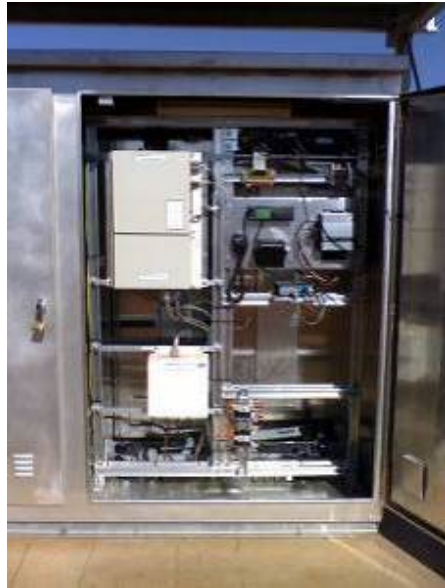
Figure 4.3 ARGUS system trackside electronics. (Inspired Systems)
