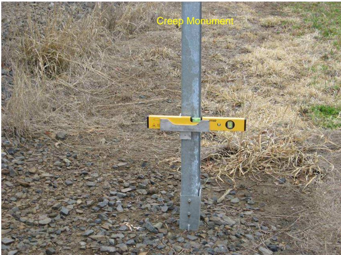
Figure 3.2 A creep monument with a spirit level that incorporates a laser.
