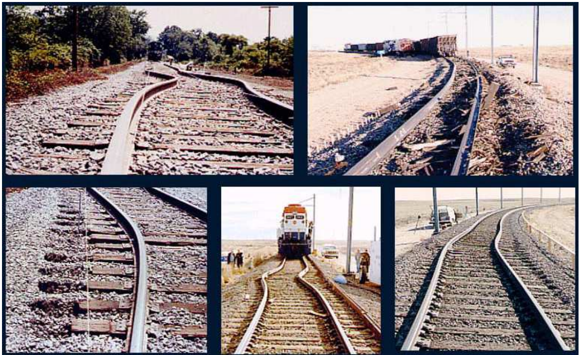
Figure 2.8 Examples of track buckling (Volpe Centre 2002)
