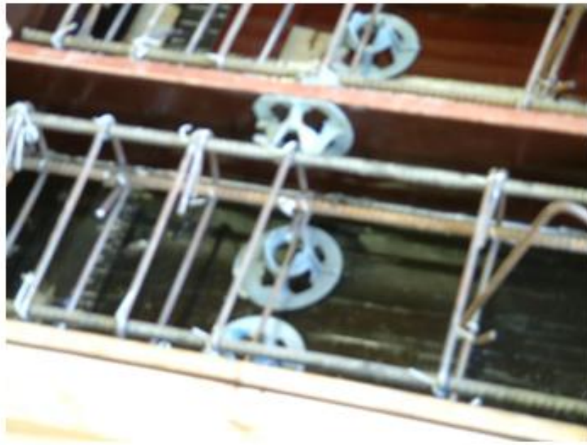
Figure 4.6: Steel Reinforcing Chairs
