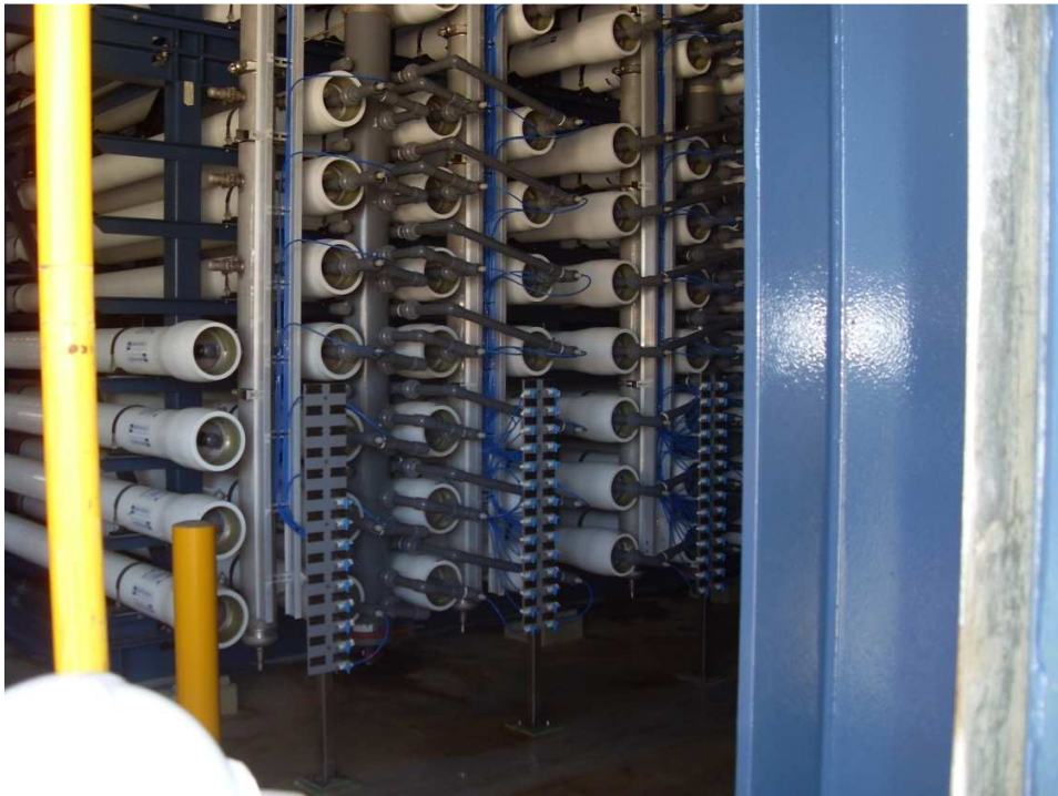
Figure 2.3.2.4 & 2.3.2.5-Vertical Sand Filters and Reverse Osmosis Membranes at the Tugun Desalination Plant, Gold Coast, Australia. Horizontal filters provide the opportunity to provide inline filtration with the RO Membranes, greatly saving on space and infrastructure costs.
