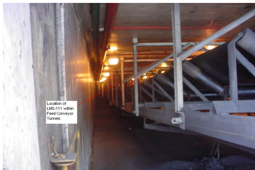
Figure 7.4: LMS-111 Location on Feed Conveyor
