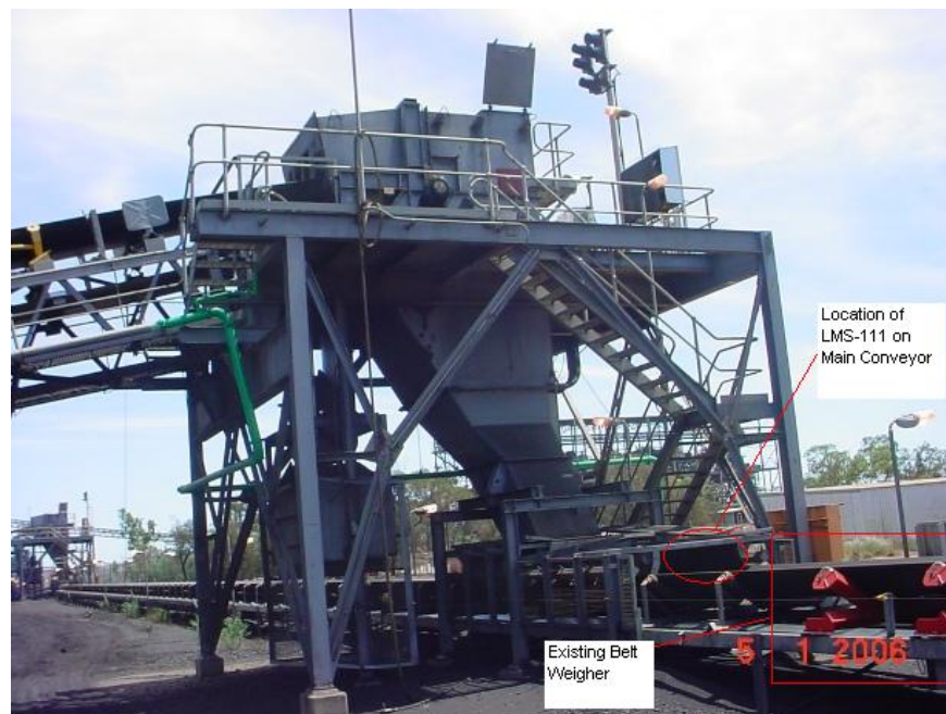
Figure 7.3: LMS-111 Located On Main Conveyor
