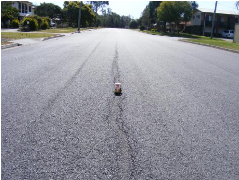
Figure 6.3: Severe pavement separation on Suffield Drive Yamanto
