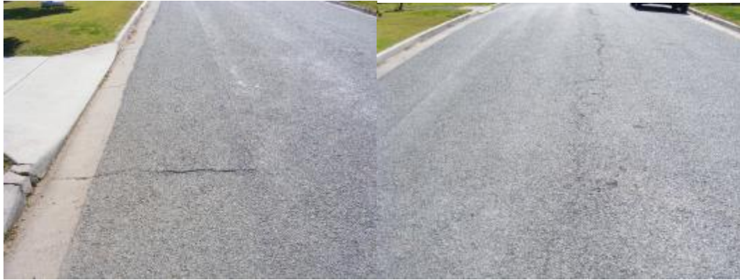
Figure 4.2: Block cracking in Phillip St
