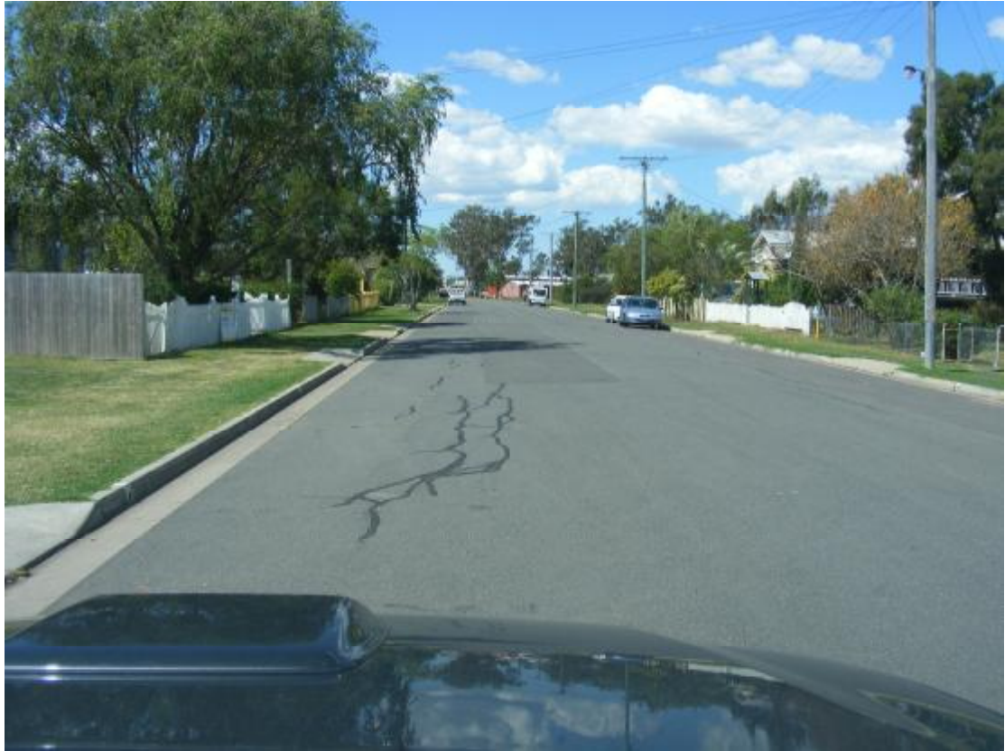
Figure 4.6: Madden Lane Rosewood longitudinal cracking
