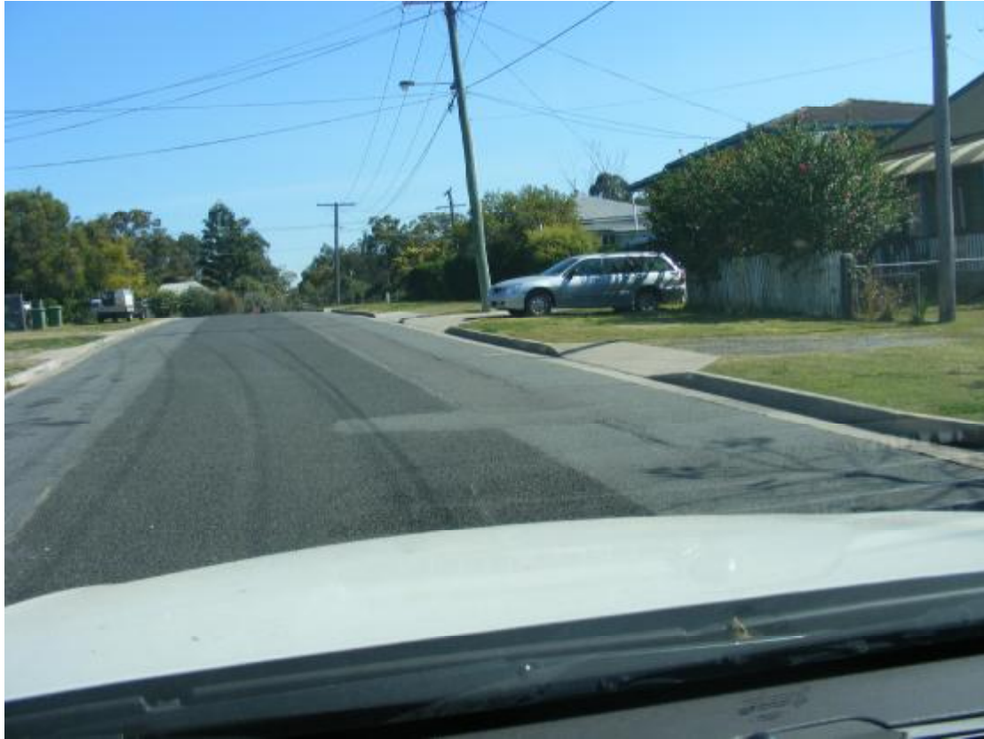
Figure 4.12: Rutting and cracking of lean mix pavement in Ross St Ebbw Vale
