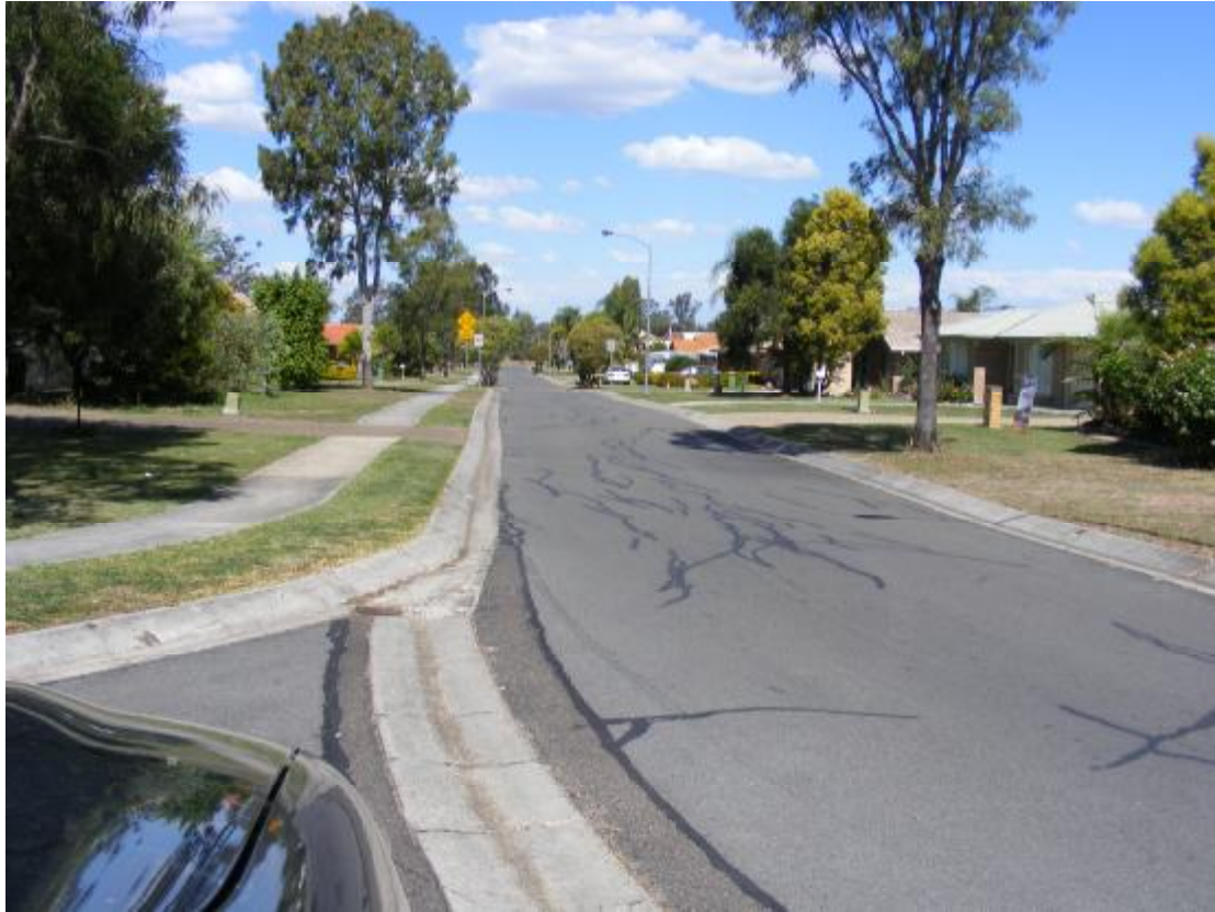
Figure 4.9: Bernadette Cres Rosewood, cracking and kerb misalignment
