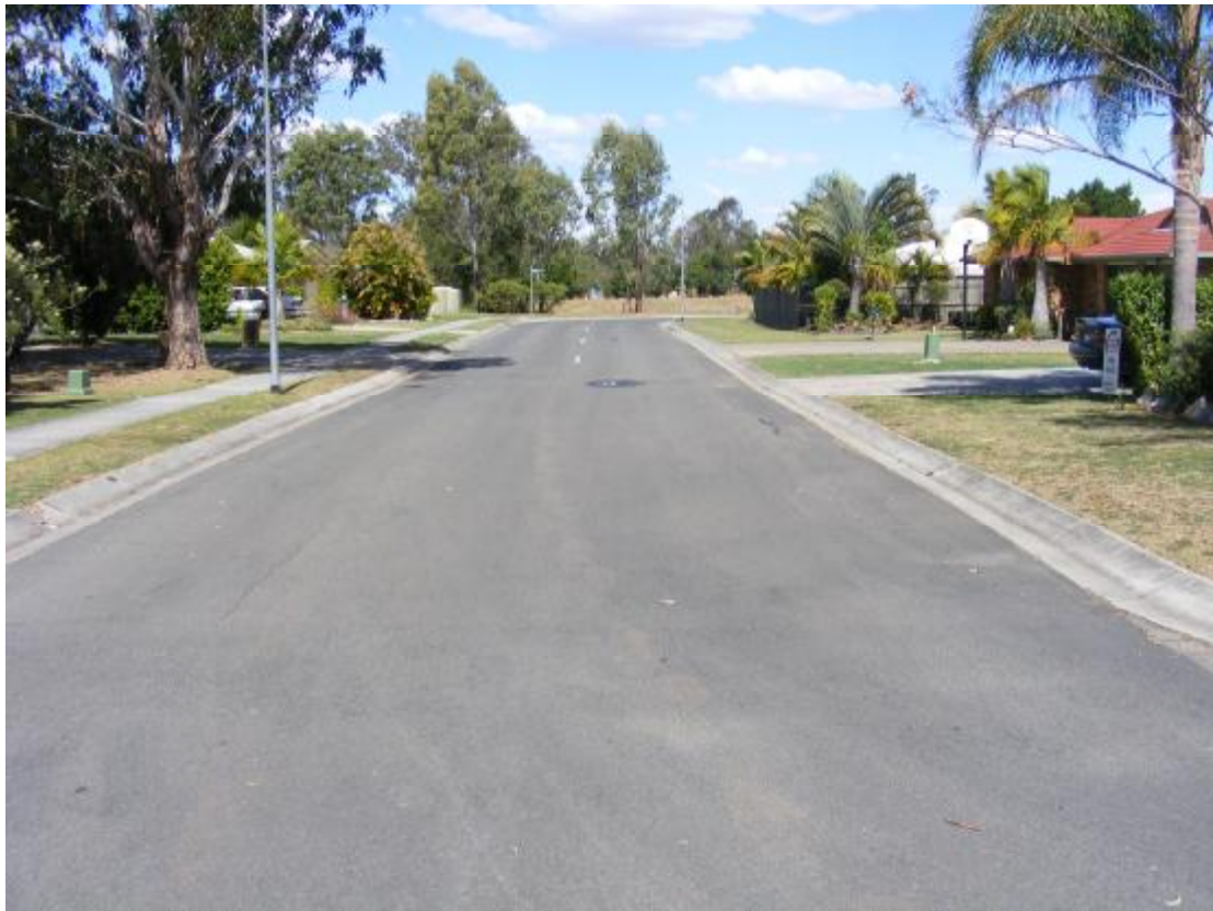
Figure 4.8: Bernadette Cres Rosewood, kerb and pavement deformation, ponding water
