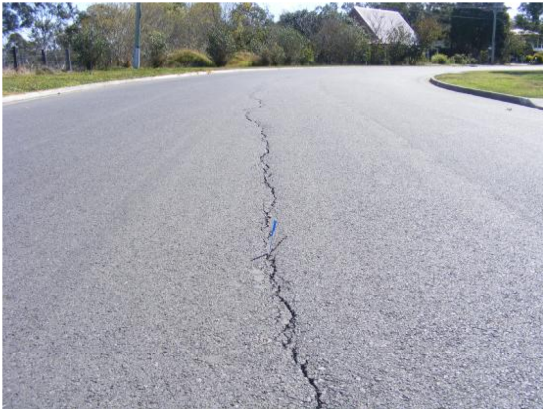
Figure 4.18: Suffield Drive section 1 longitudinal cracking
