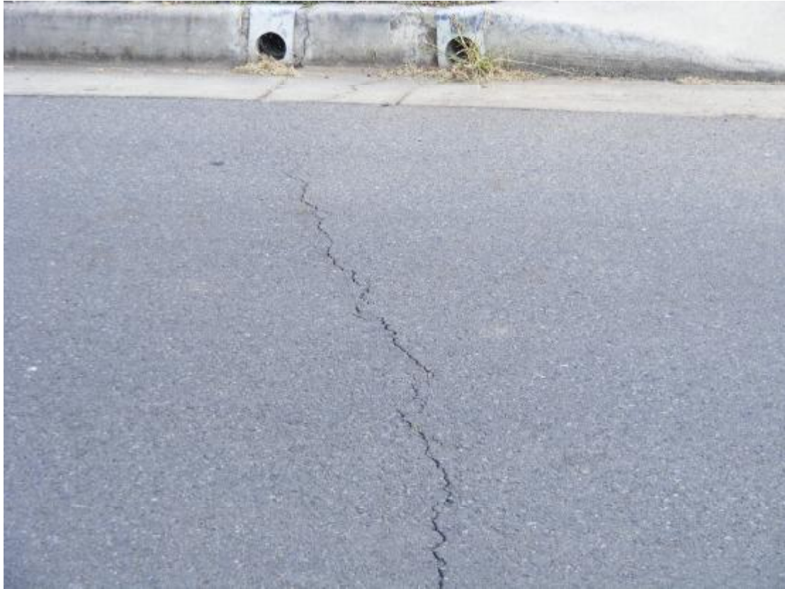
Figure 4.16: Close up view of block cracking in Margret Street
