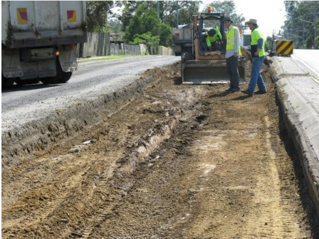
Figure 8.1: Soft subgrade on Redbank Plains Road
