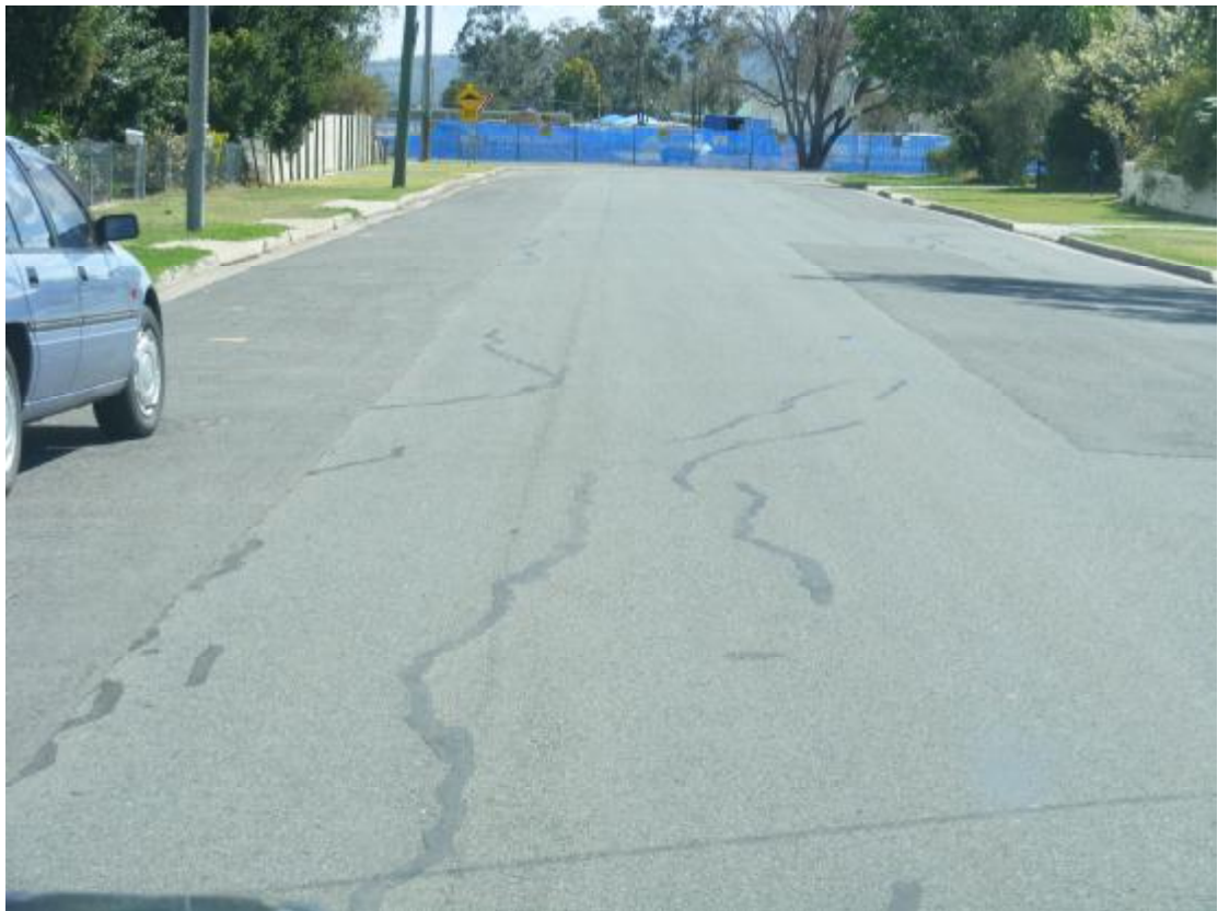
Figure 4.7: Madden Lane Rosewood failures and cracking
