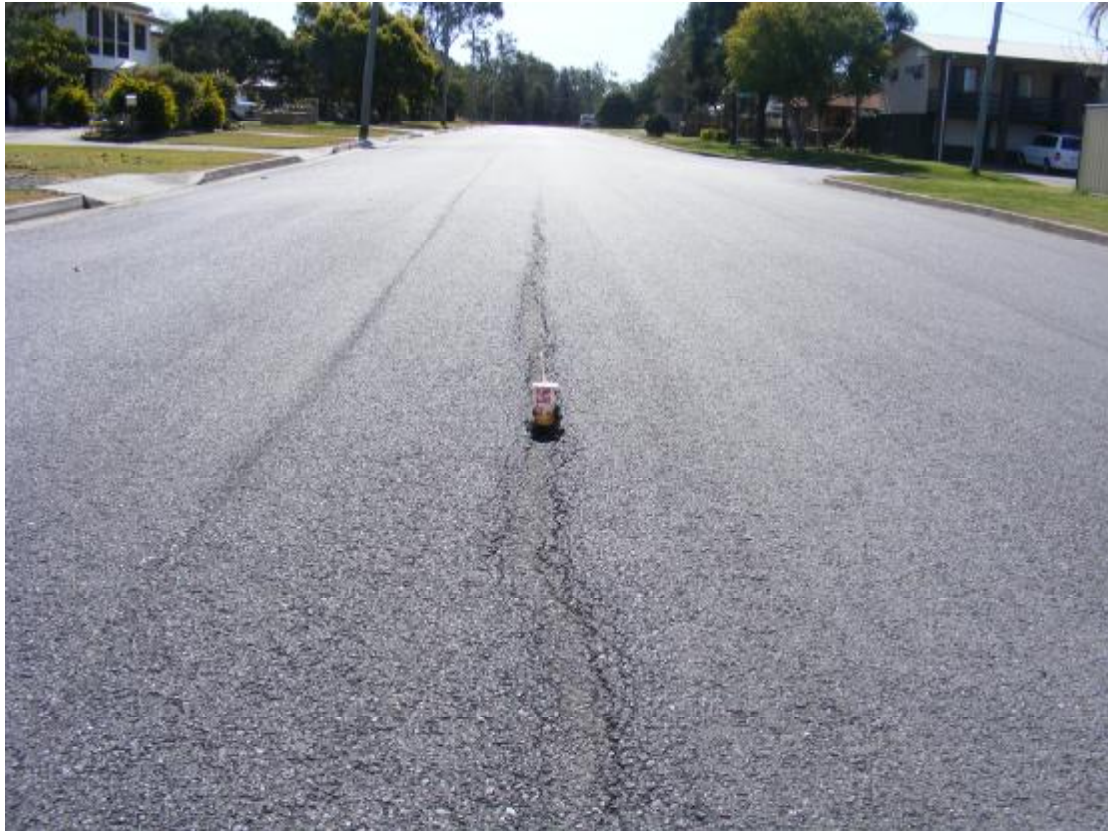
Figure 4.19: Suffield Drive section 1, cracking large enough for a coke cup
