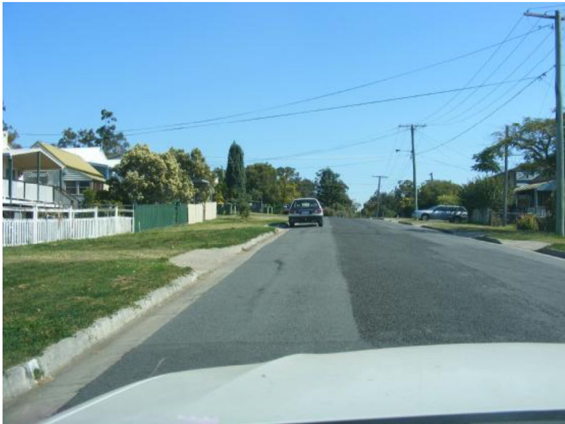
Figure 4.11: Rutting of lean mix pavement in Ross St Ebbw Vale
