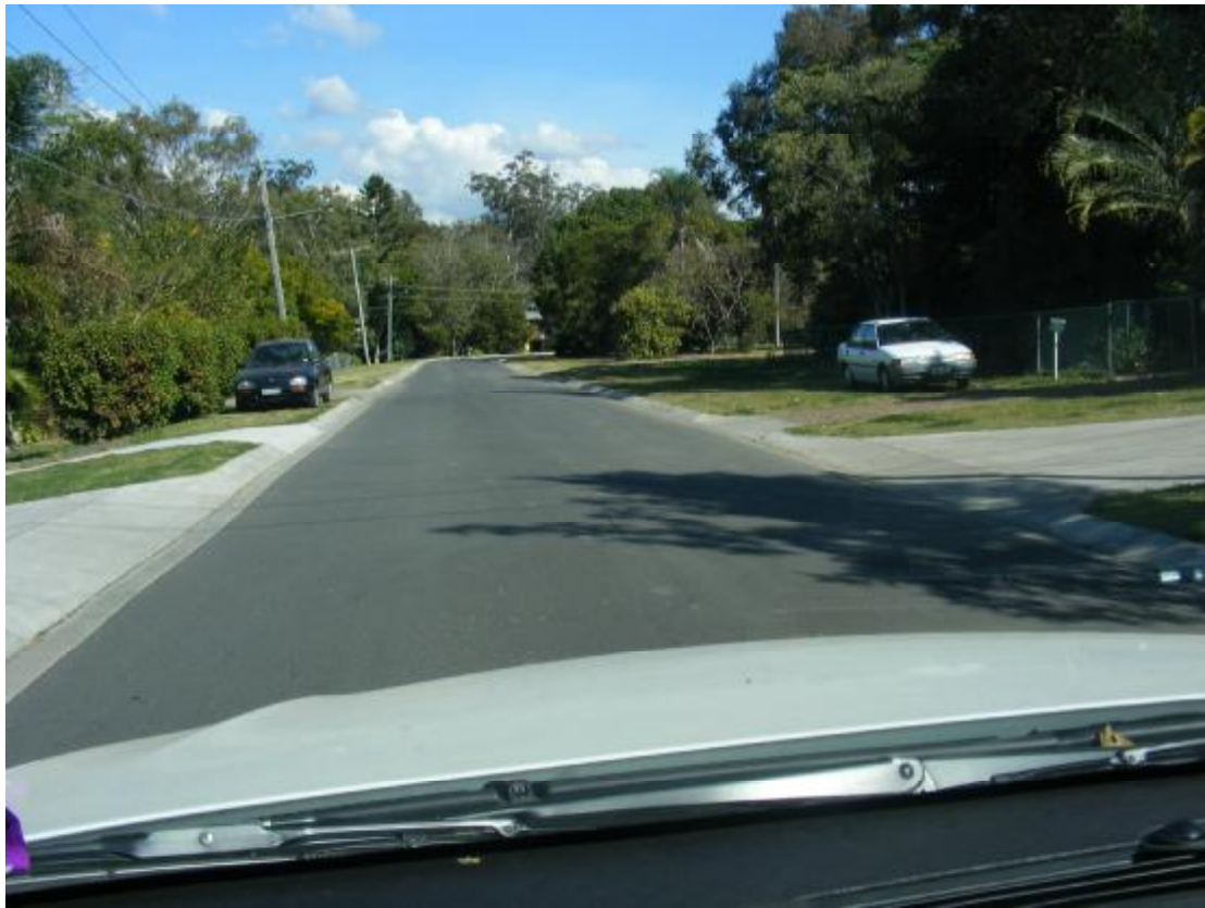
Figure 4.13: distant view of Boscawan Cres showing crack over gas main
