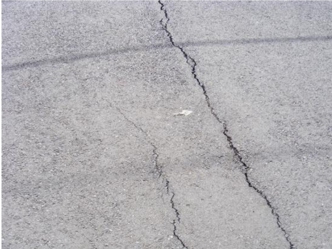
Figure 4.14: Close up view of Boscawan Cres showing crack over gas main
