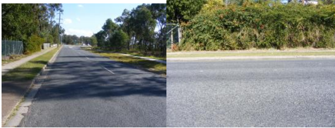
Figure 4.5: rutting deformation on Brennan Street Bellbird Park.
