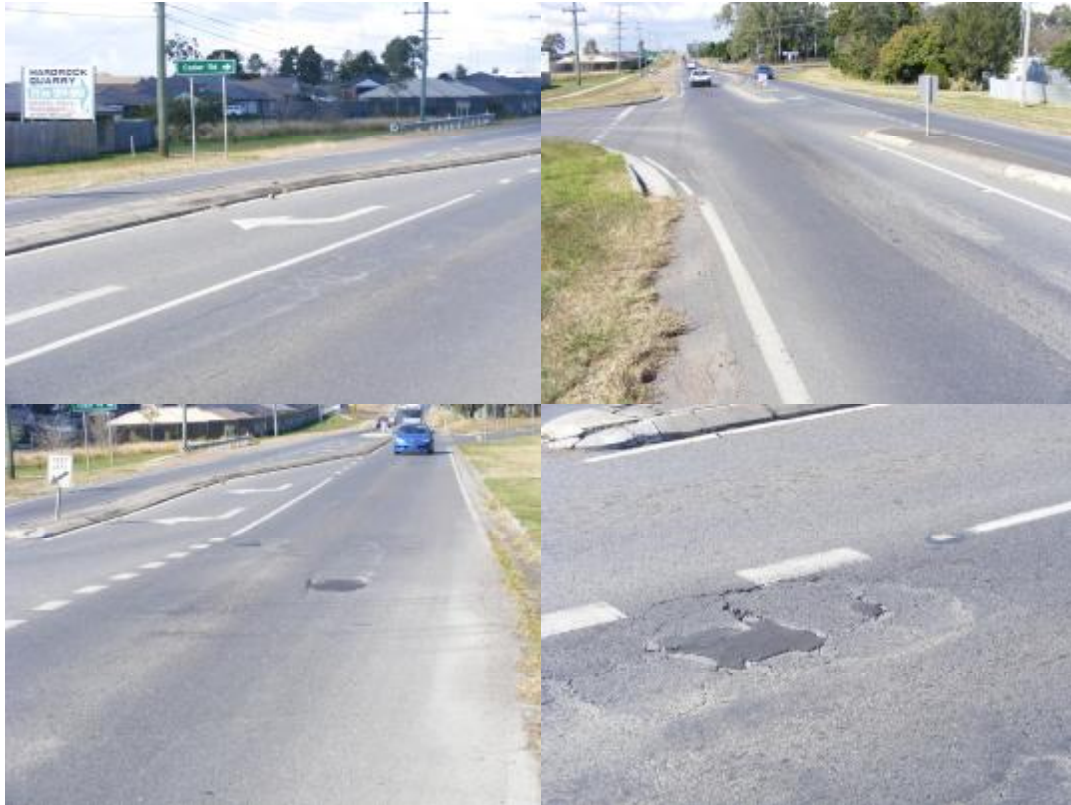
Figure 4.4: Bad rutting and cracking on Redbank Plains Road
