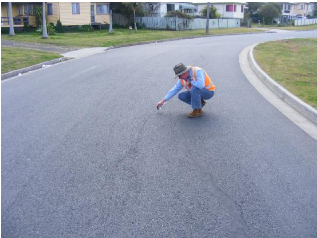
Figure 4.15: Cracking in Margret Street large enough to fit a key down.
