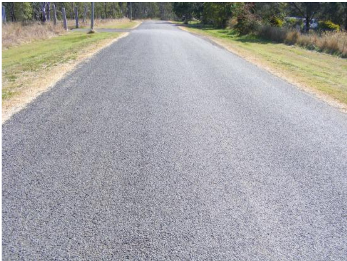
Figure 4.20: Suffield Drive section 2 perfect condition
