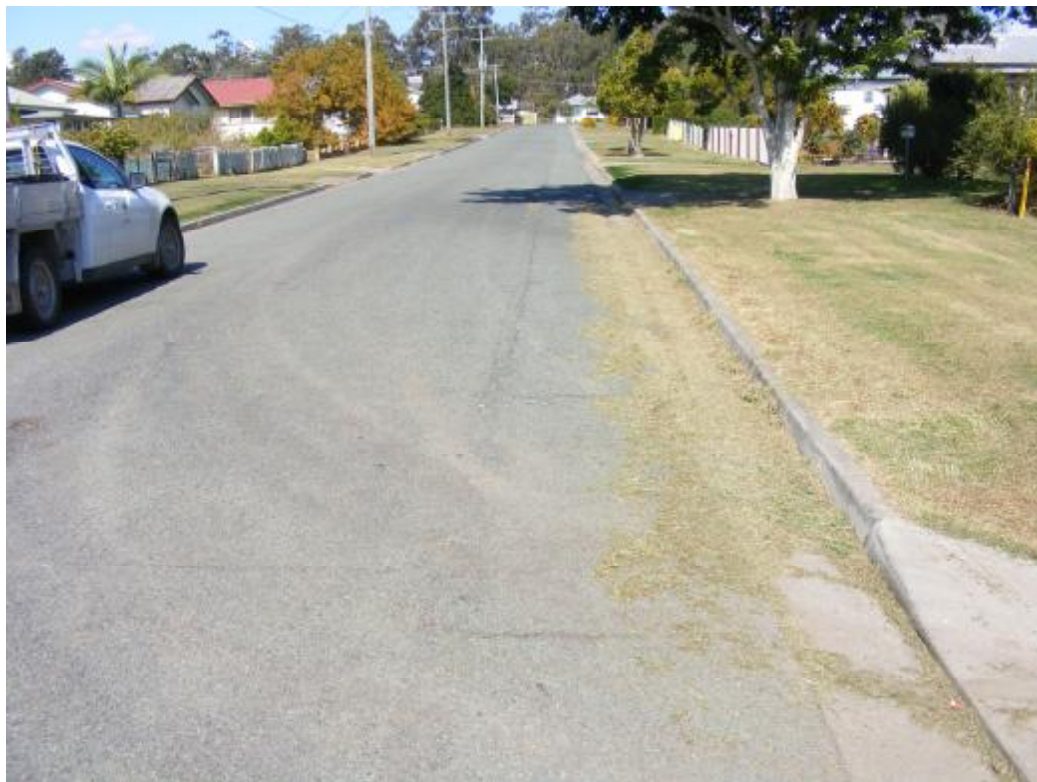
Figure 4.1: Lean mix widening reflective cracking on Phillip St
