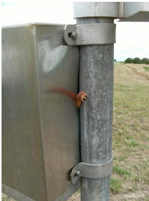
Figure 8.1: A broken or cut meter cable
