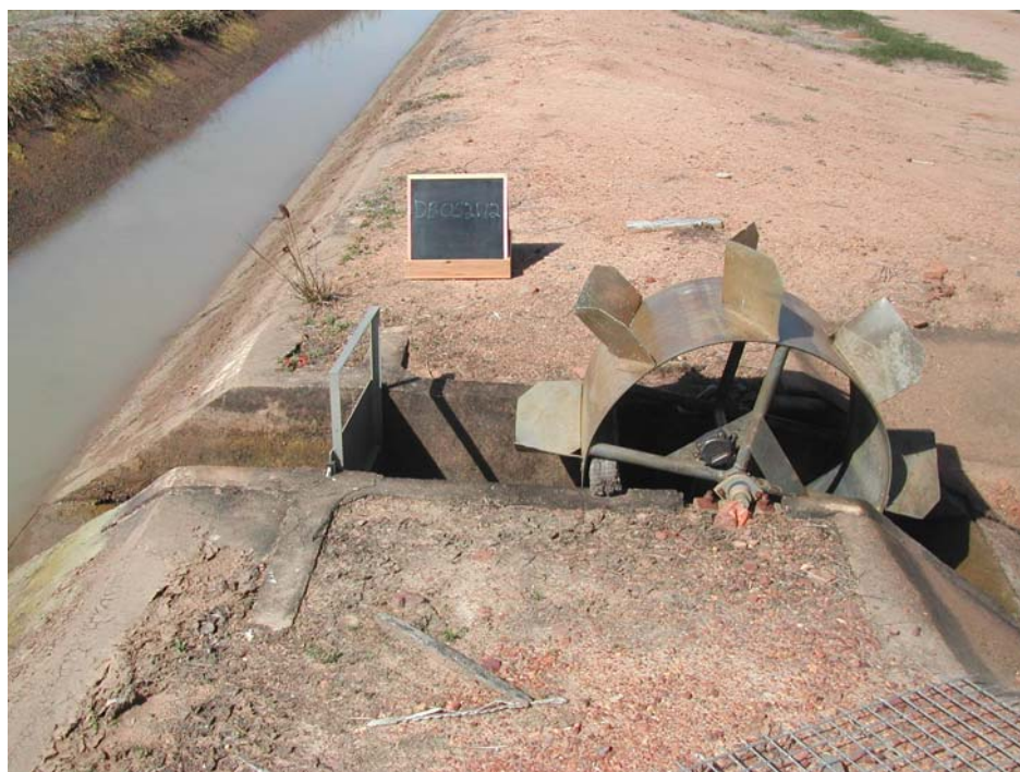
Figure 6.1: A Dethridge Wheel
