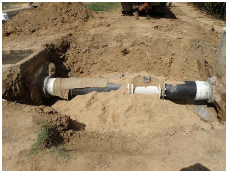
Figure 4.4: A recent Electromagnetic Meter installation
