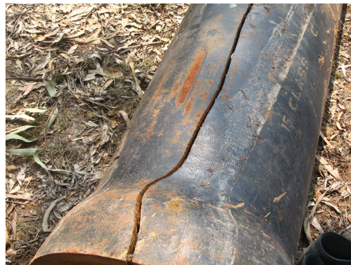
Figure 2.10 Longitudinal Split in a Cast Iron Pipe
