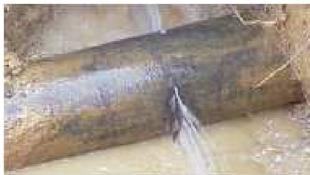
Figure 2.9 Circumferential Break in a Cast Iron Pipe (WSAA 2003)
