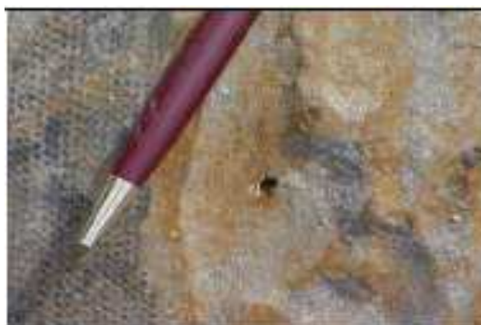
Figure 2.12 Pinhole Leak in a Ductile Iron Pipe (WSAA 2003)
