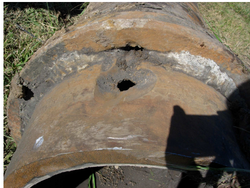
Figure 2.13 Joint Failure Caused by Perished Lead Joint
