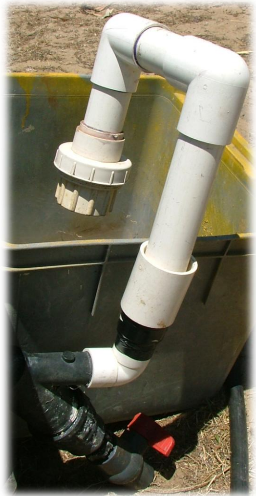
Figure 4-12: Overflow and drain valve
