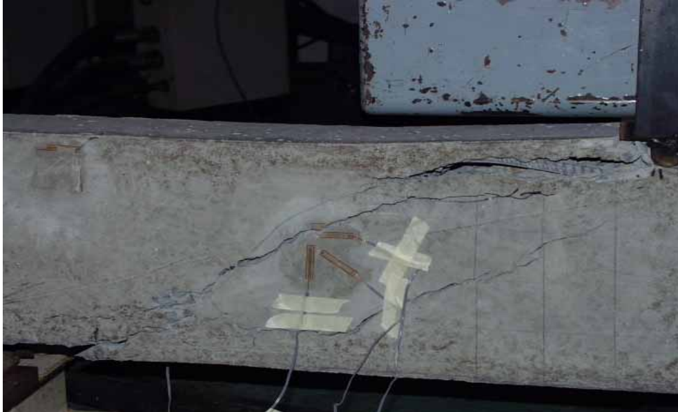
Figure 5.7: Failure Crack Pattern of Beam B1
