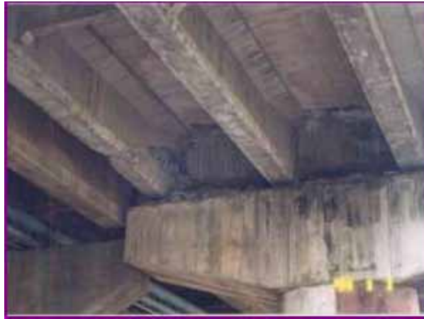
Figure 2.1: Crack in Girder
