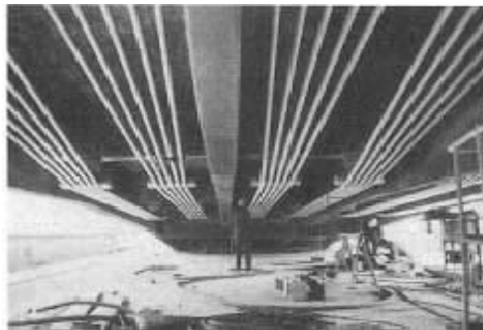
Figure 2.4: Bridge at Aue: External Prestressed bars of the drop-in span (Source: VSL report series, 1999)
